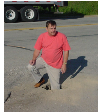
Figure 3: Improper pothole restoration
