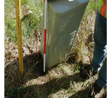
Figure 1. Pedestal too close to R/W pin.
