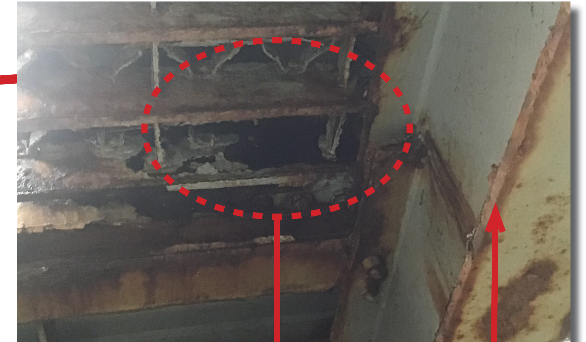
Severe Deterioration under Median Barrier Corroded Stringer
