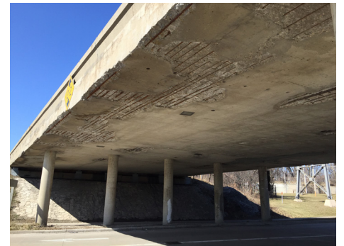
Deteriorating bridge conditions
