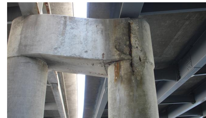
Deteriorating bridge pier at I-94 bridges over 70th Street
