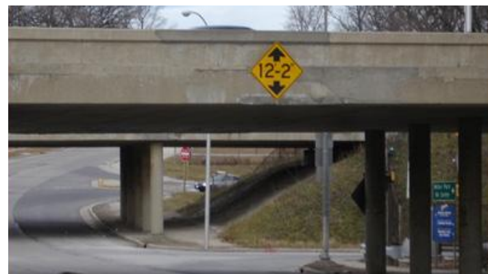
I-94 bridge over Mitchell Boulevard. Due to the low clearance of this bridge, several trucks crashed into the underside of the bridge and became stuck. The incidents have contributed to the deterioration of the bridge.
