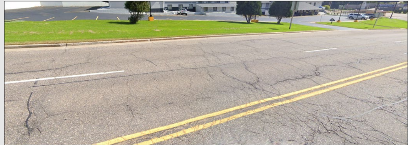
US 12 Pavement Deterioration
