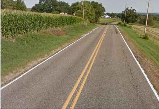
WIS 113 pavement rutting
