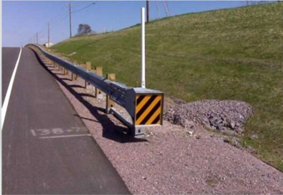
Energy Absorbing Terminal (EAT)
