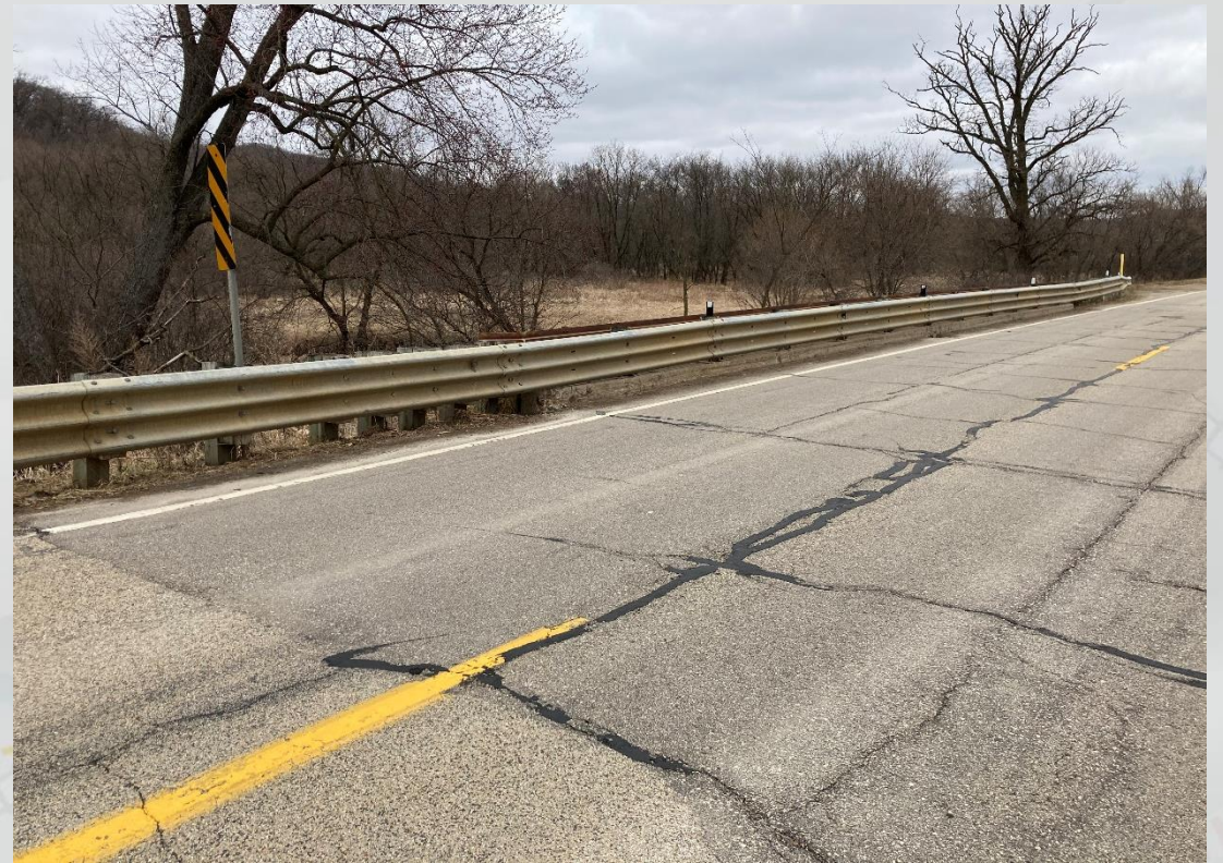
WIS 130 Block Cracking
