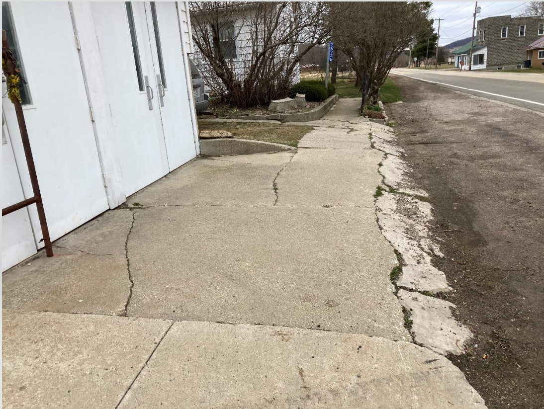
Sidewalk deterioration in Bear Valley
