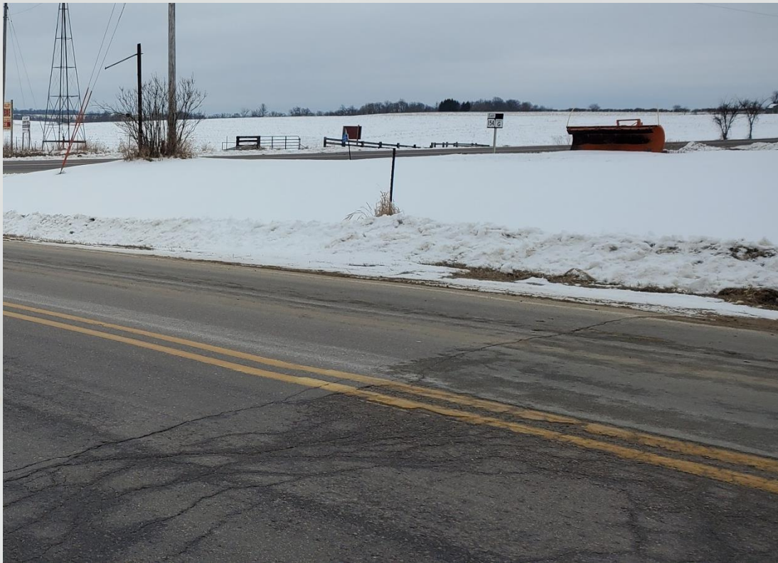
WIS 130 Alligator Cracking
