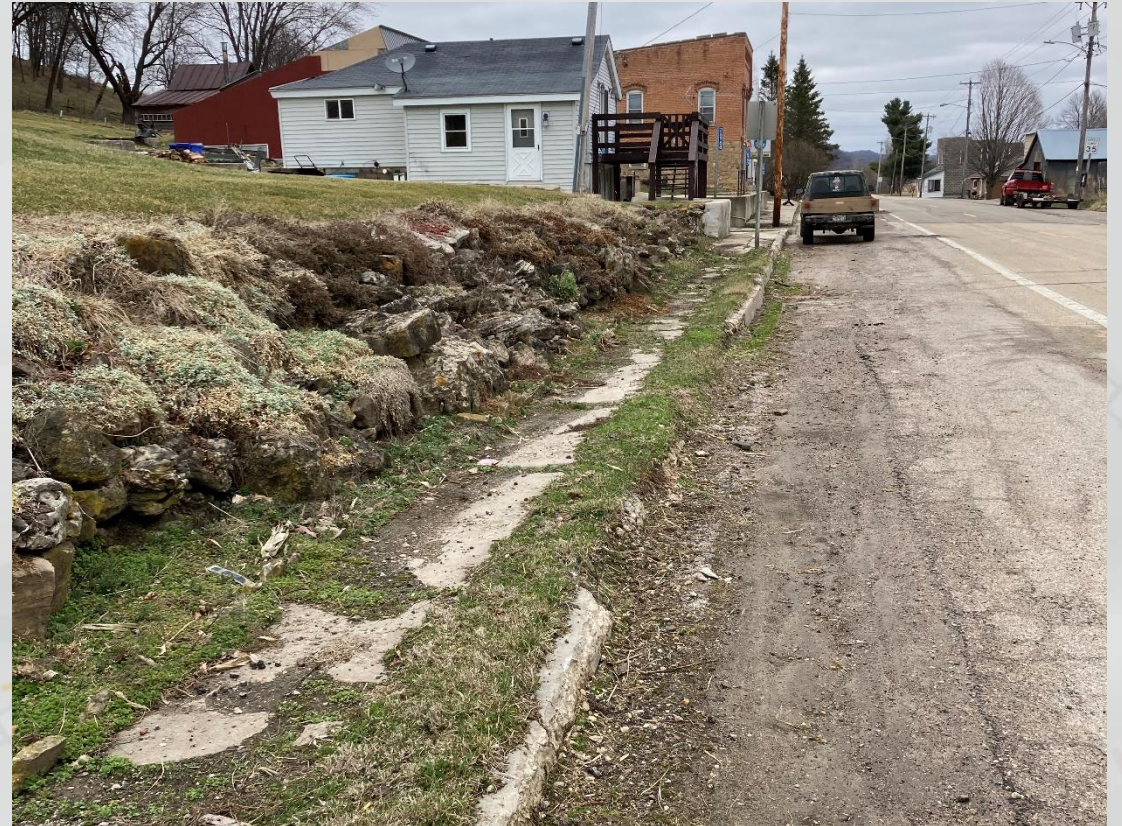
Deteriorated Curb & Gutter in Bear Valley
