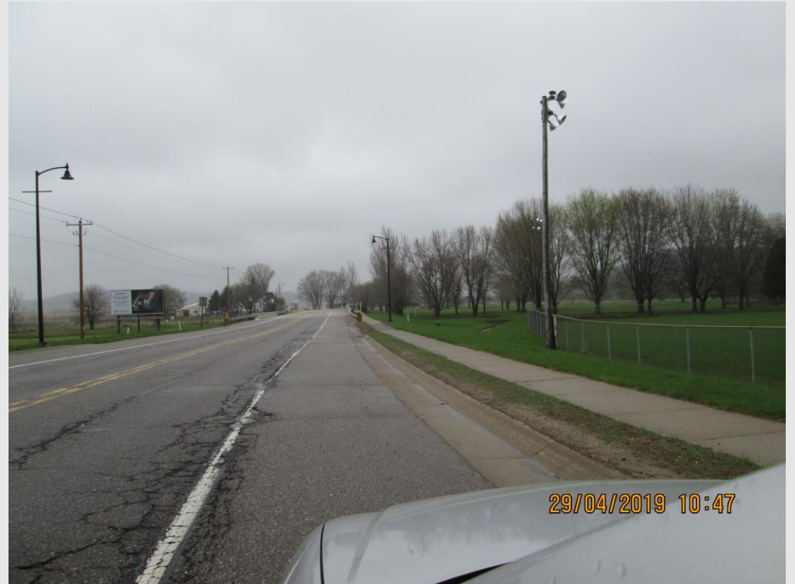
WIS 23 Pavement Cracking
