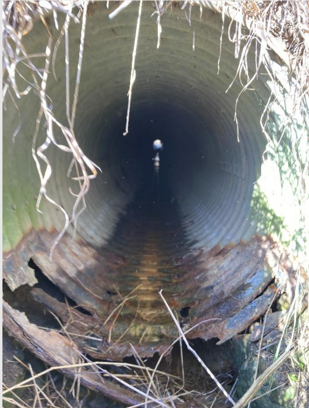
Culvert Pipe – Poor Condition
