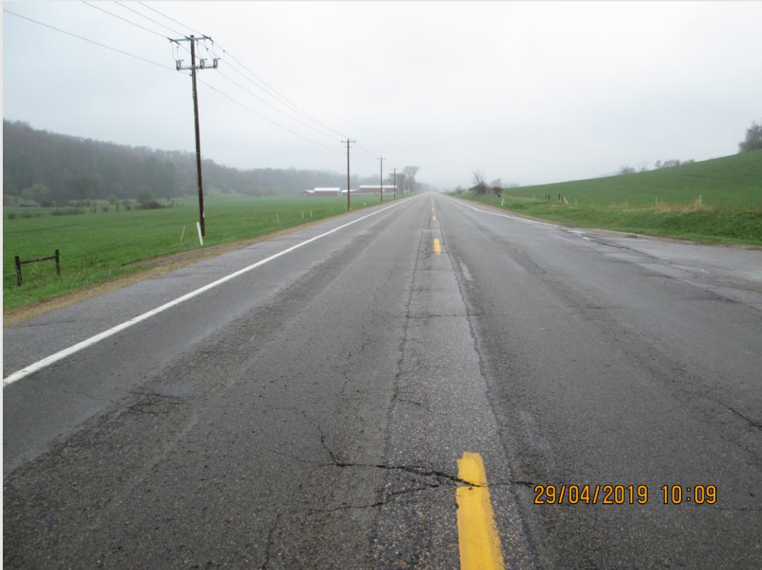
WIS 23 Pavement Rutting
