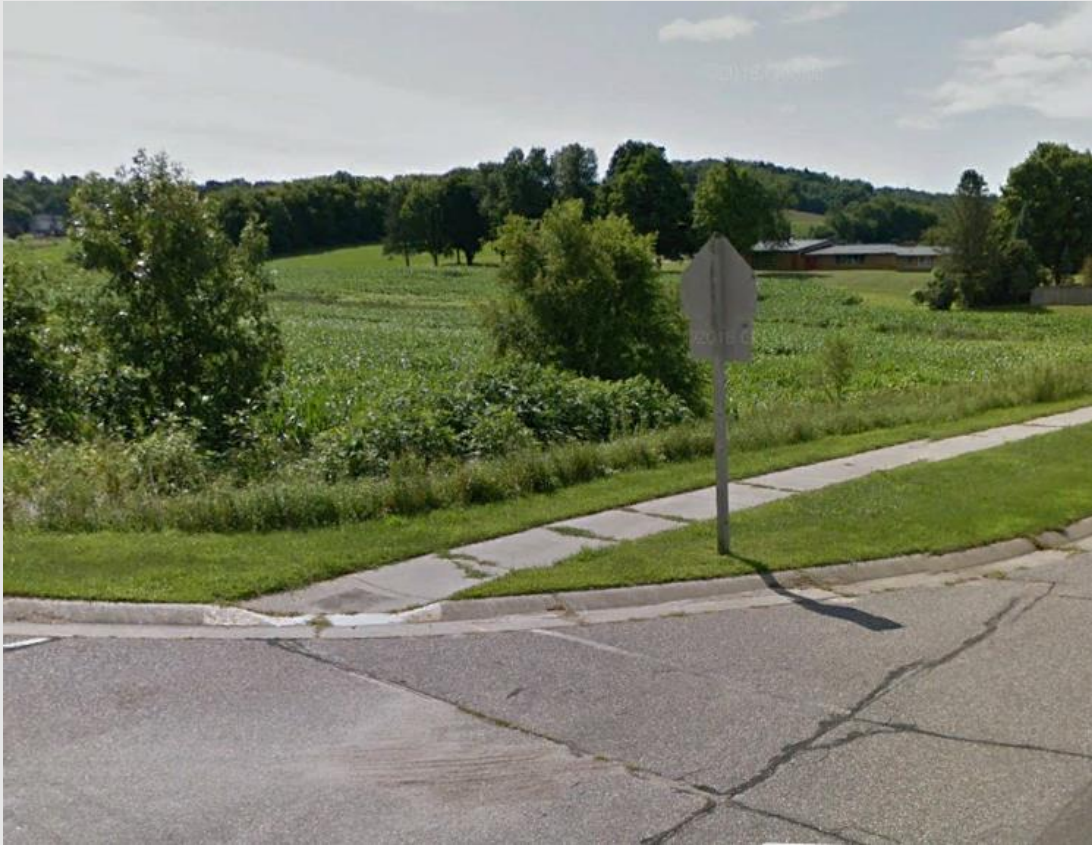
Non-ADA Compliant Crosswalk
