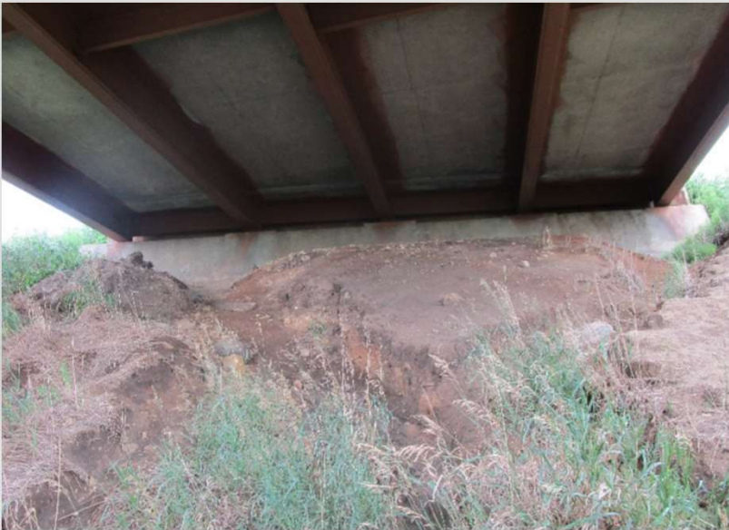
Slope Erosion under B-11-66
