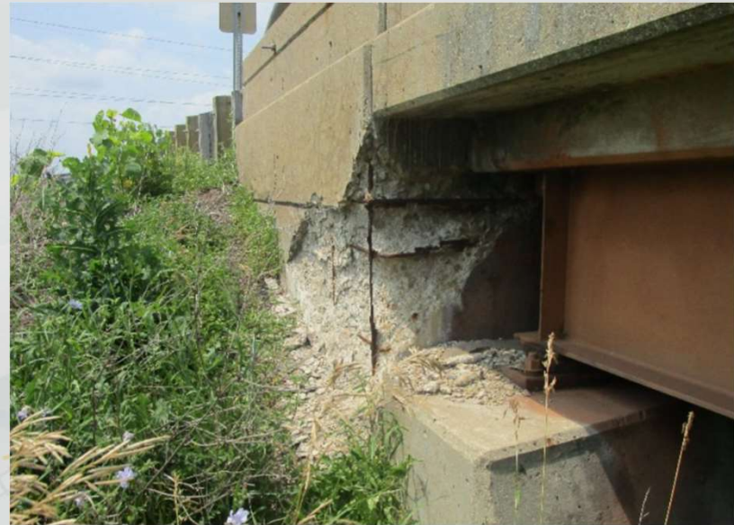
Exposed Rebar on B-11-66
