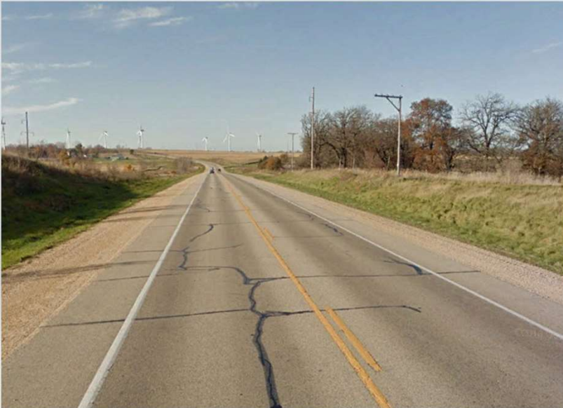
WIS 33 Pavement Rutting
