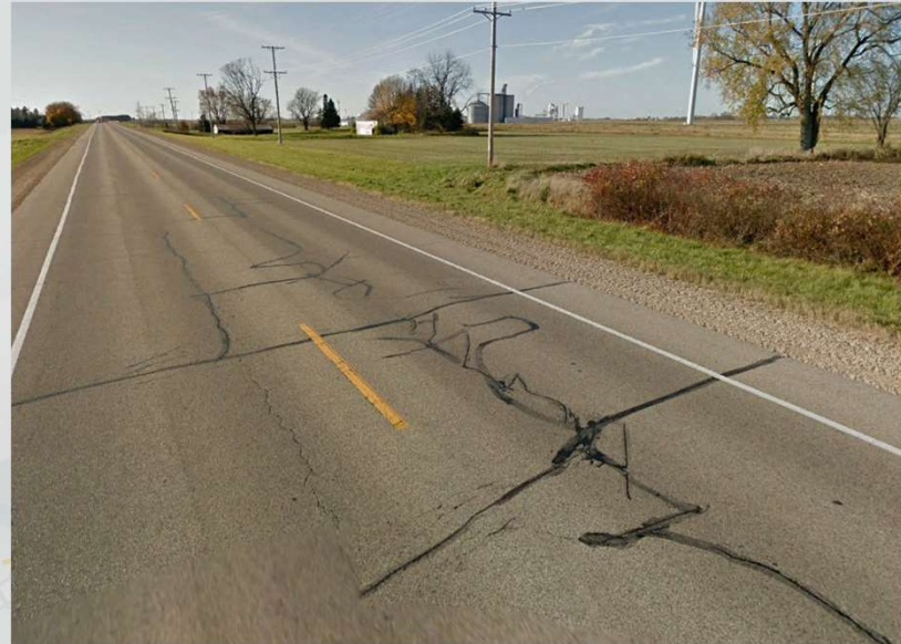
WIS 33 Pavement Cracking
