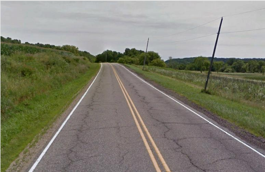
WIS 58 Alligator Cracking Urban Areas
