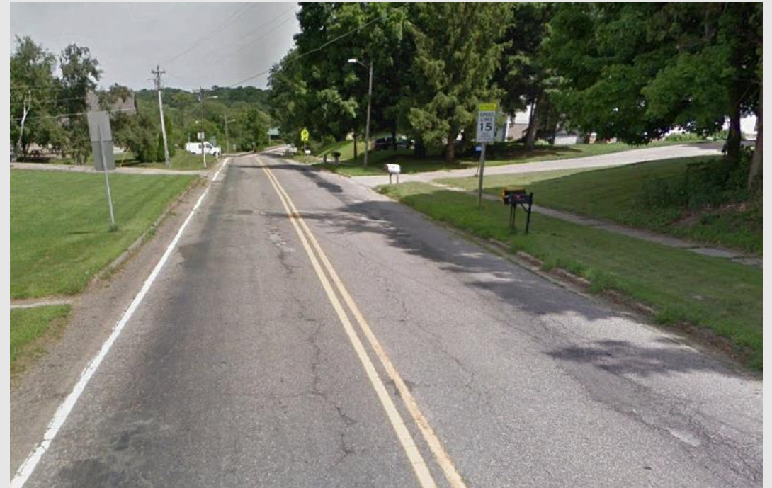
WIS 58 Alligator Cracking and Rutting in La Valle
