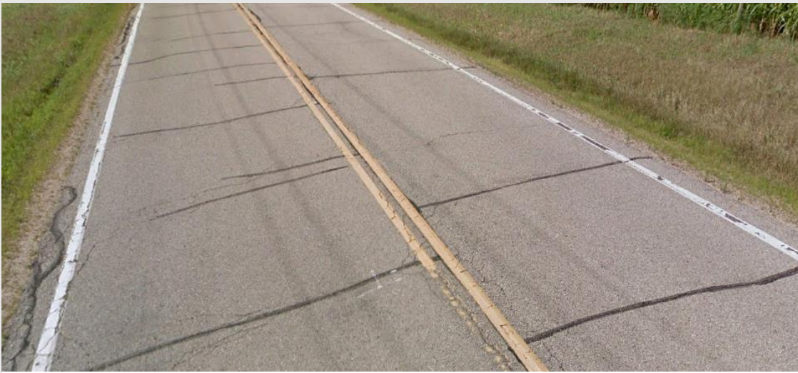
WIS 78 pavement cracking
