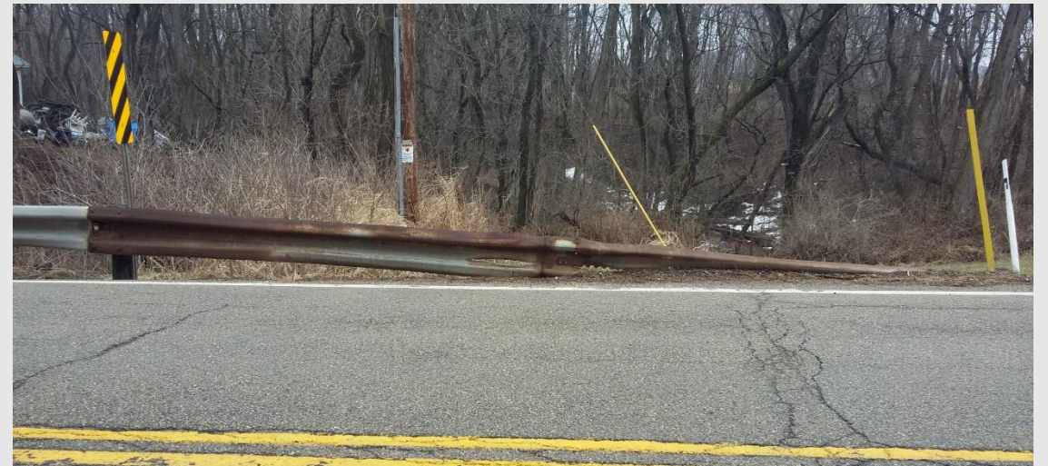
Existing end of guardrail on WIS 78
