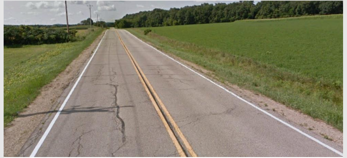
WIS 78 pavement cracking
