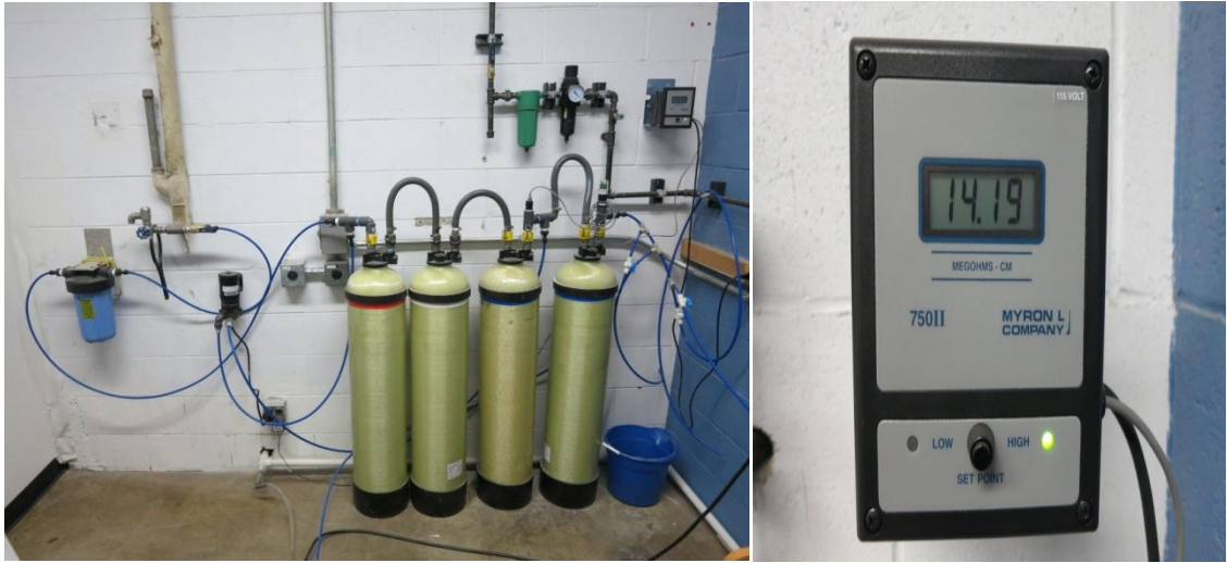
Figure 21: Water Purification System and Mega Ohm Meter
