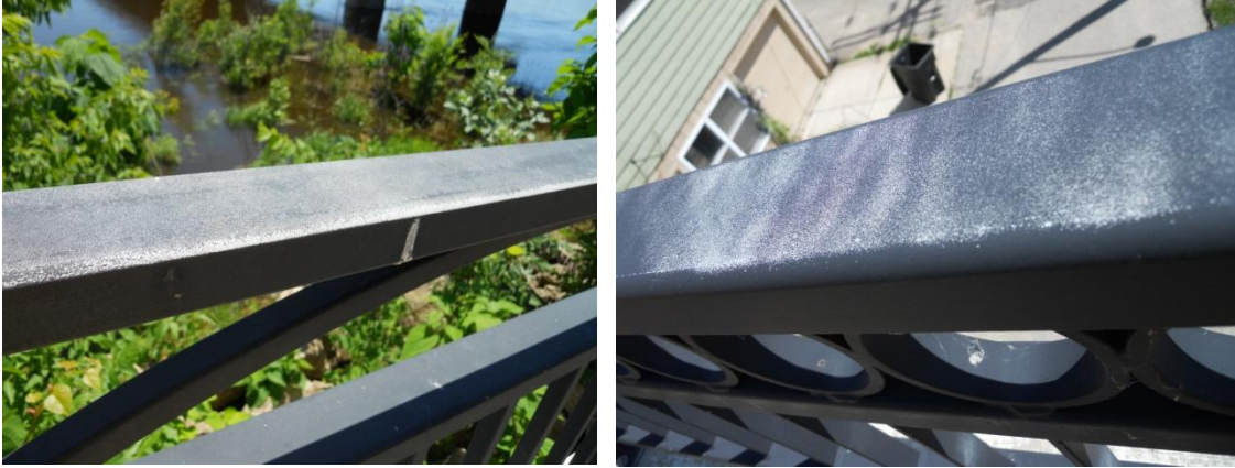
Figure 9: Jefferson Bridge Railing Exposed Tie-Coat
