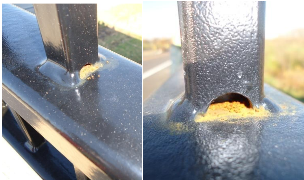
Figure 14: Highland Ave and I-43 Bridge Railing Corrosion
