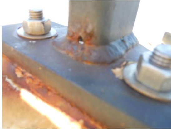
Figure 8: Sauk City Bridge Railing Drainage Hole
