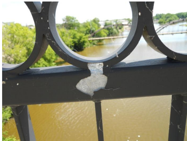
Figure 10: Jefferson Bridge Loss of Adhesion in Railing Coating
