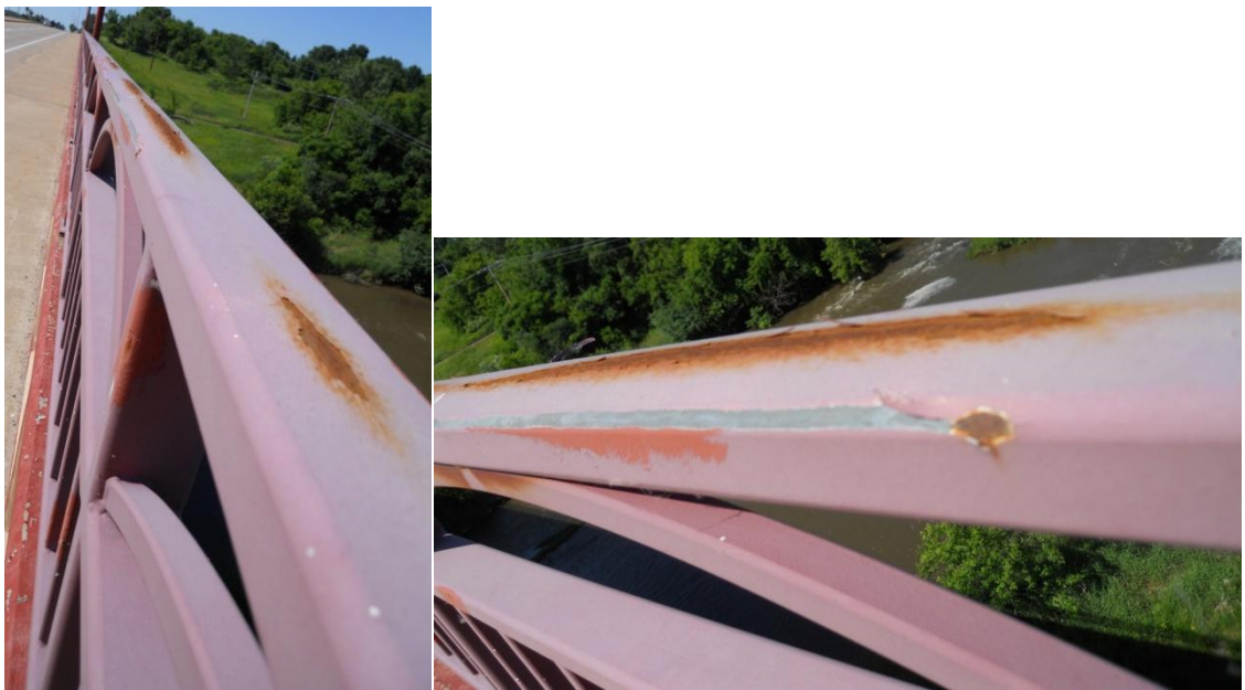
Figure 5: Baraboo Bridge Railing Damage Due to Freezing
