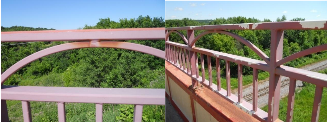
Figure 3: Baraboo Bridge Railing Top-Coat Failure
