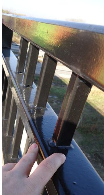
Figure 15: Highland Ave and I-43 Bridge Railing Blocked Vent Holes
