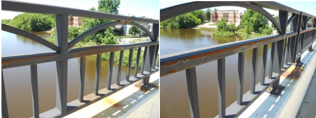
Figure 7: Sauk City Bridge Railing Damage Due to Freezing
