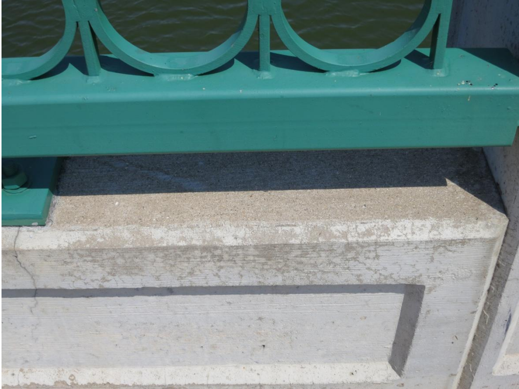
Figure 0-3: Loss of coating film on horizontal surface and the immediately adjacent vertical surface of a parapet.
