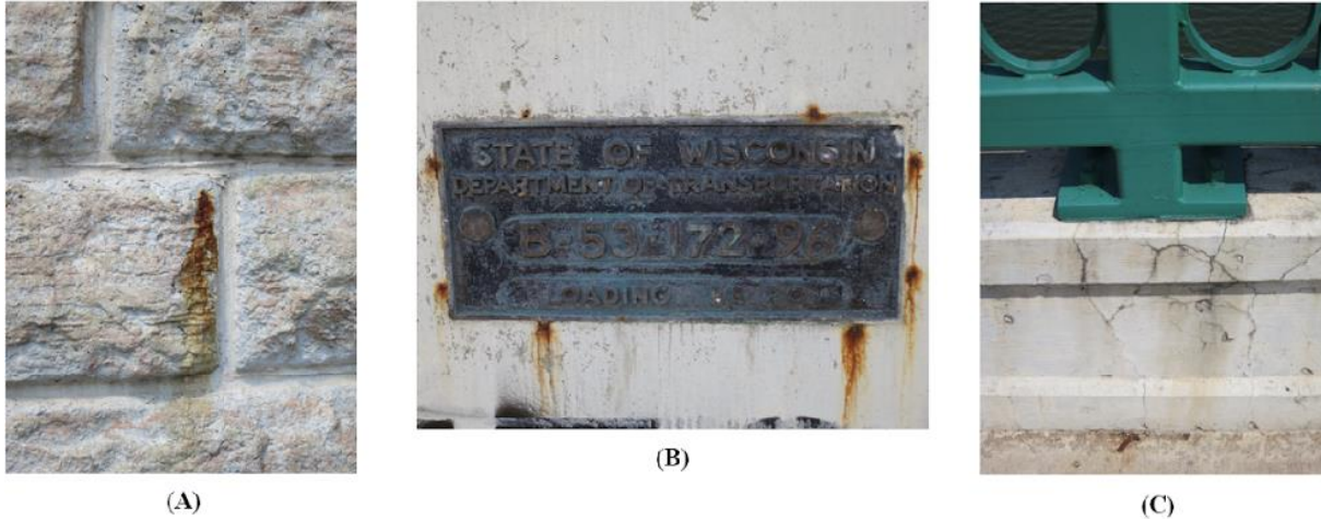
Figure 0-4: Examples of rust staining; (A) Exposed reinforcement on form lined surface, (B) Surrounding structural identification plaque, (C) Cracking near anchoring of steel guardrail.
