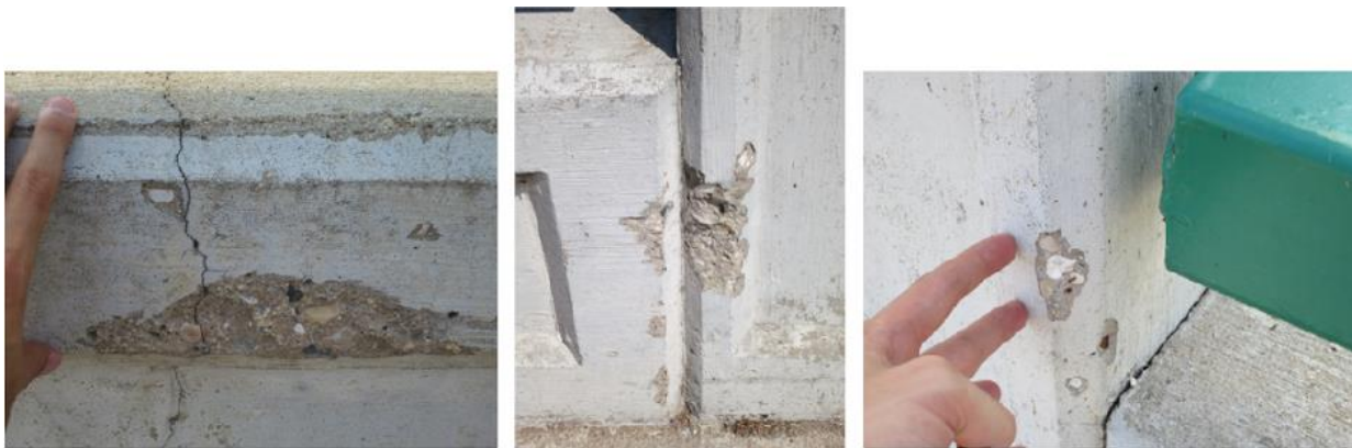
Figure 0-5: Examples of spalled concrete on the Portland Avenue Bridge (Beloit, WI).
