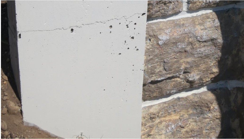
Figure 0-2: Discontinuities in coating film caused by surface voids.
