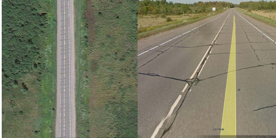
Figure 4-25 Satellite and street view photos from Google Earth ® of the distresses (SN 14300)
