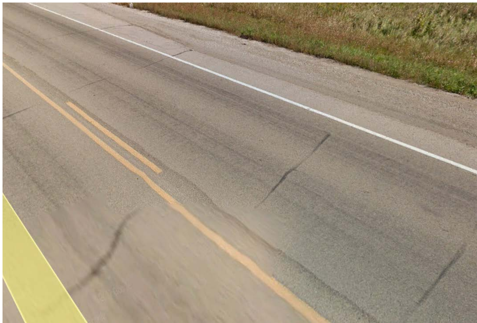
Figure 4-50 Pavement condition on the place with the highest compaction variation (SN=60850)
