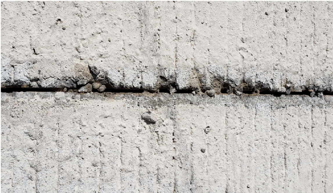
Figure 2.5.10: Aggregate Dislodgement Noted on Sawing from Previous Day
