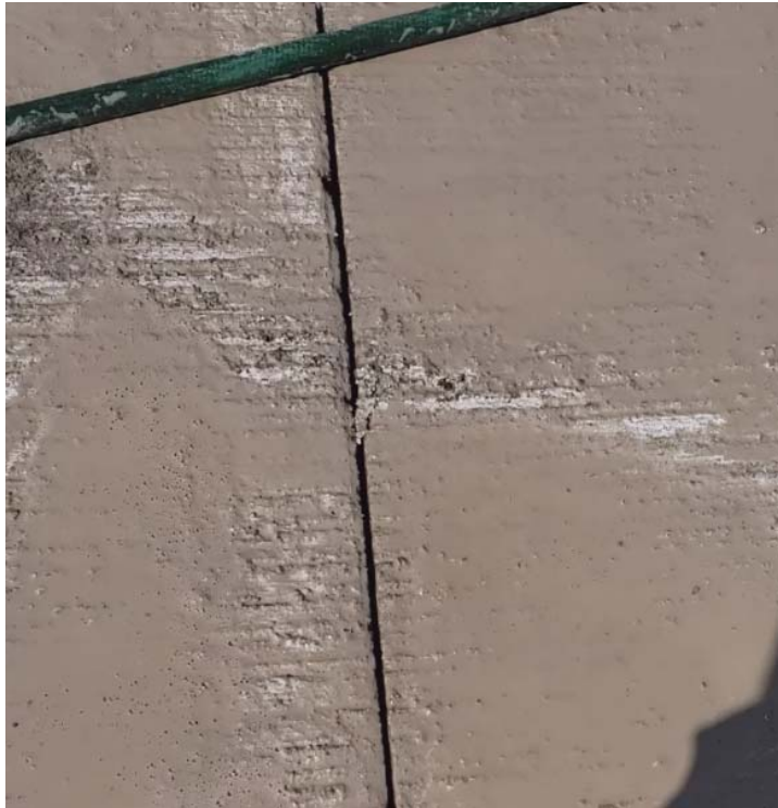
Figure 2.5.9: Joint Crack Due to Wheel Movement
