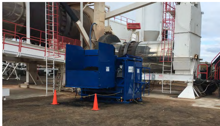
Dry crumb rubber addition system at plant
