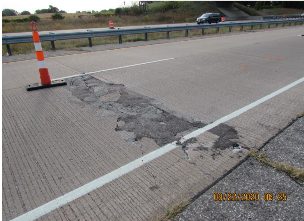
Figure 2. Recently buckled joint on I-39 SB in Columbia county, WI.
