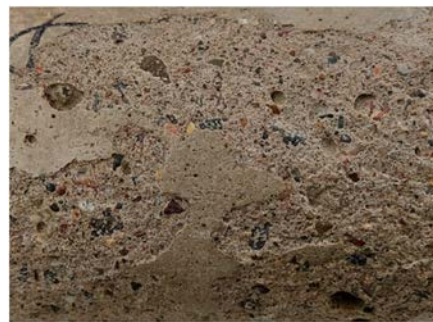
(b) PCC surface scaling
