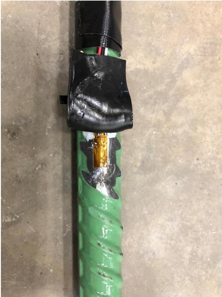
Figure D.4. Strain gage installed on reinforcement adhesively anchored into lower wingwall.
