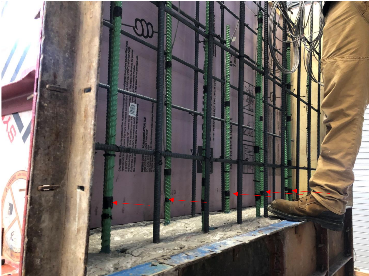
Figure D.5. Photo showing location of strain gages (red arrows) on reinforcement anchored into lower wingwall prior to casting of upper wingwall concrete.
