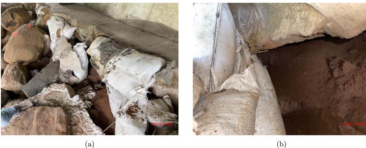
Figure 34: B-58-075 a) Concrete slurry repair with sand bags left in place attached to the repair and adding dead weight due to soil erosion under repair, b) Scour under the abutment
