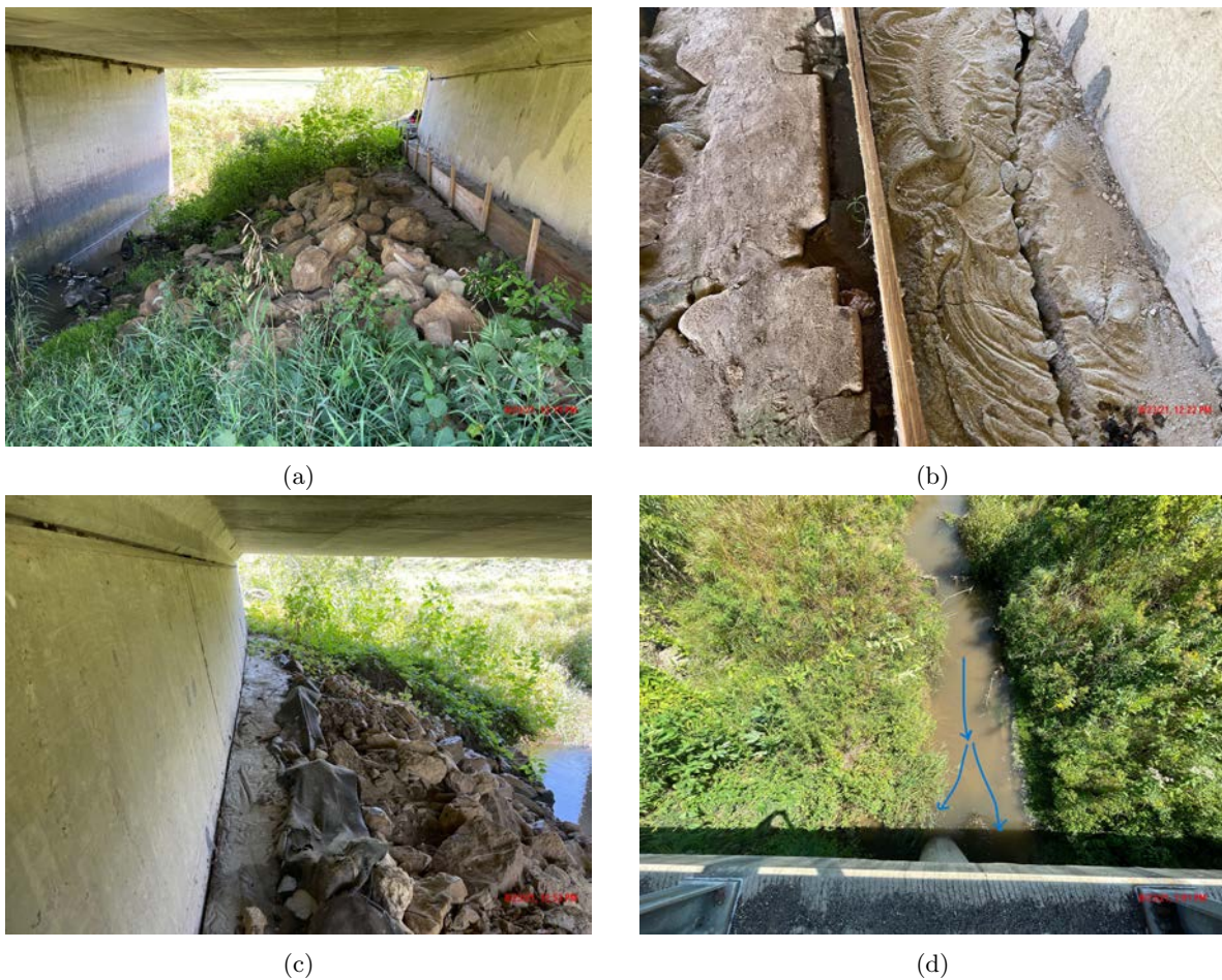
Figure 15: B-52-114 a) South abutment, overall view, b) Zoomed in photo of wide crack in closure pour, c) North abutment concrete pour repair noted with a gap between the abutment and pour repair indicating movement of repair. Abutment stem (typical for both abutments) is 8 degrees out of plumb inwards towards the pier, d) Upstream at center pier. Blue arrows indicate water flow.
