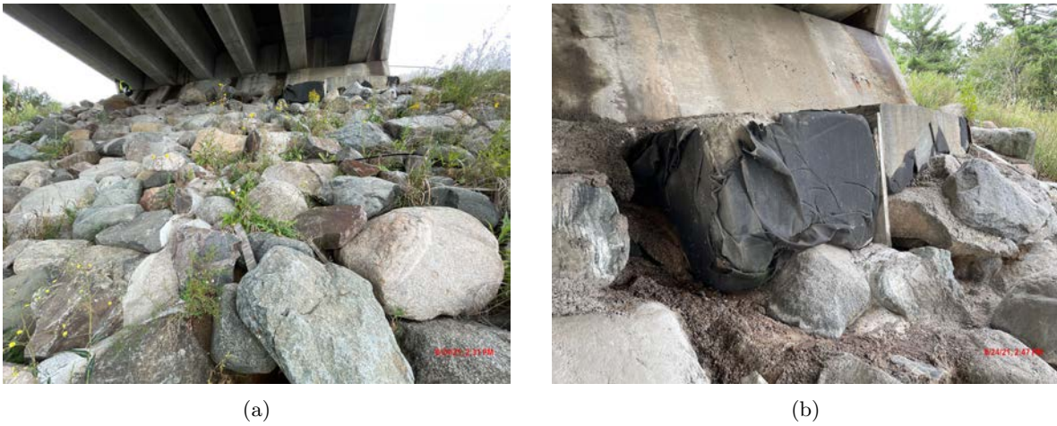
Figure 23: B-35-063 a) North abutment overall, b) Riprap repair near east end of north abutment
