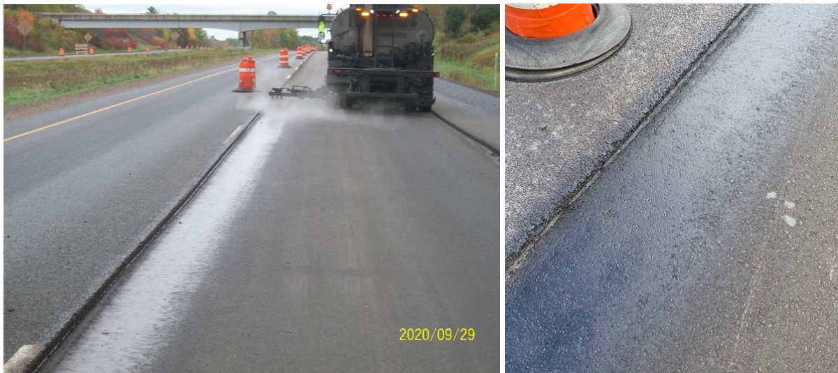
Figure 18. RPE remedial application to low joint density area (left); after penetration and drying (right). Author photos.
