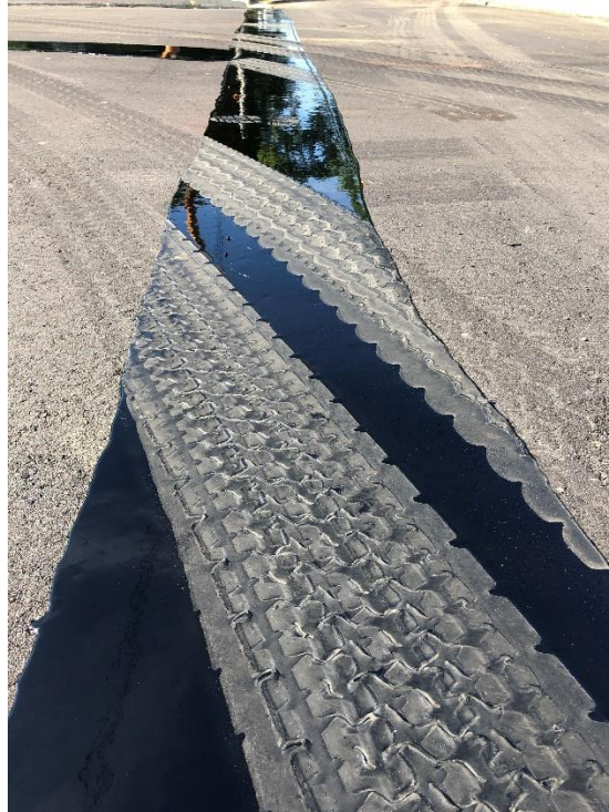
Figure 13. VRAM tracking resistance showing some dust contamination from truck tires. Author photo.
