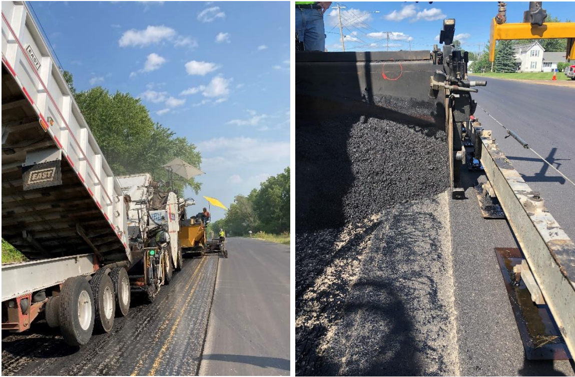
Figure 14. Placing hot-side pass on tack coat against a milled out vertical joint (left) and on a notched wedge joint (right); State Highway 22, August and September, 2020. Author photos.
