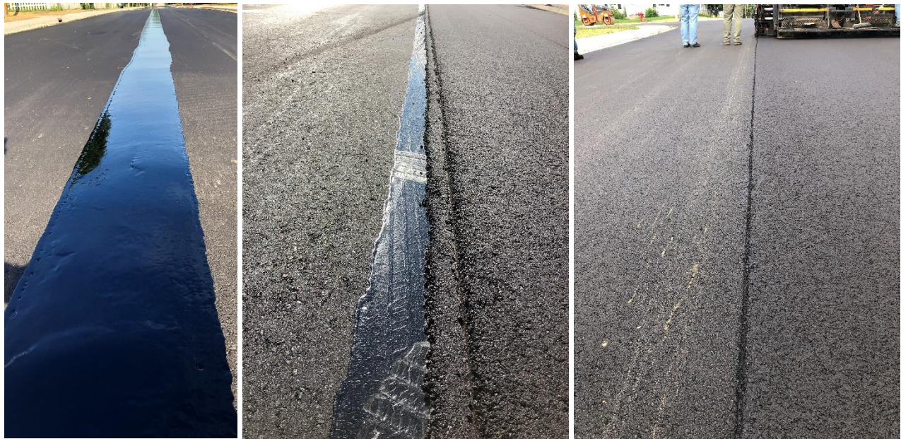
Figure 12. VRAM applied to existing surface before paving (left); VRAM after placing first pass (center); final pass before rolling (right). Author photos.
