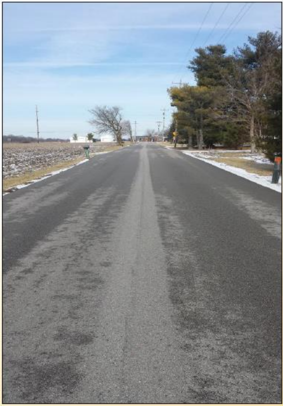
Figure 17. Treated joint during Spring melt event showing water resistance (19)
