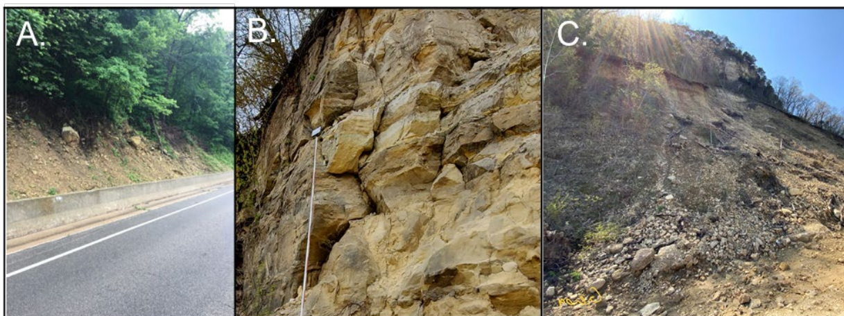
Schematic 2-6. Representative photos for each of the three hazard mechanisms identified along the study corridor. A. Rockfall sourced from the upper colluvium (typically dislodged boulders that are >1yd 3 ). B. Fragmental rockfall and rockslides sourced from the Jordan Sandstone. C. Shallow colluvial slides in the upper colluvium and lower colluvium/Lone Rock Formation.
