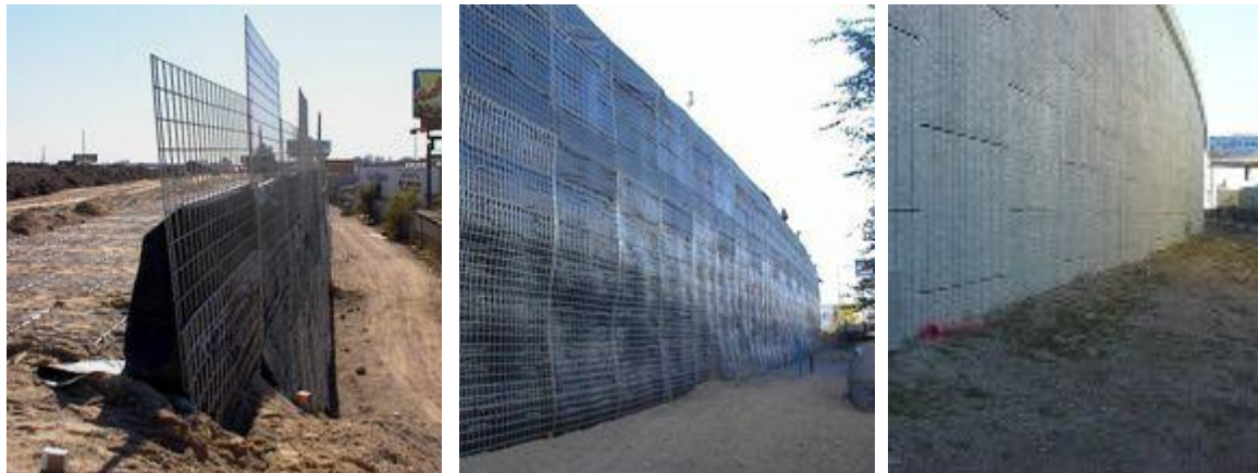
Figure 29. Photographs of the MSE wall constructed at 3600 south and I-15 in Salt Lake City-Utah (Budge et al., 2006)
