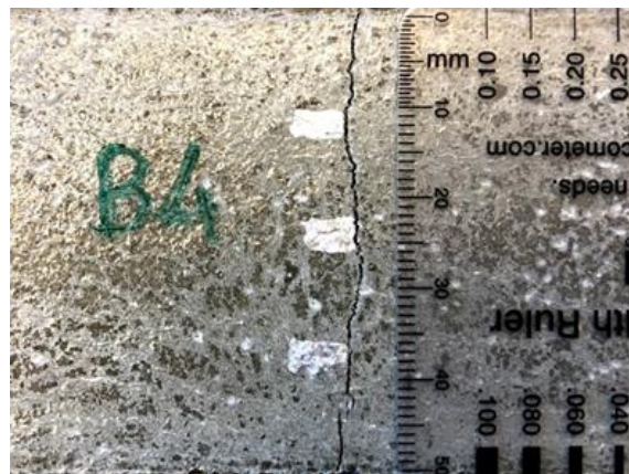
Figure 10 - Shrinkage cracking in an example test specimen.
