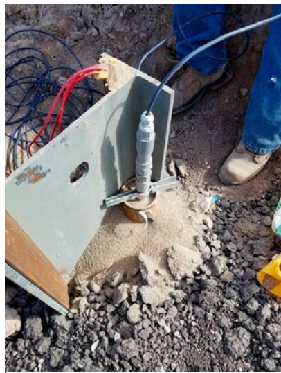
A Shaped Array Accelerometer secured at ground level.
