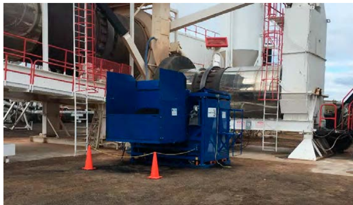
Dry crumb rubber addition system at plant
