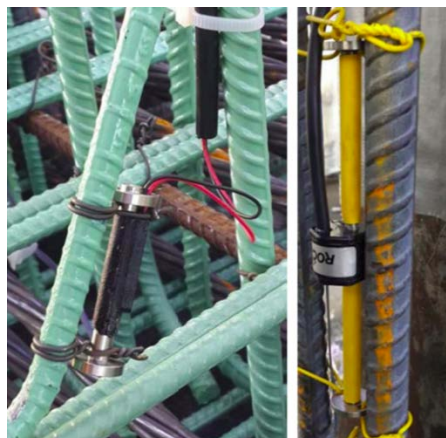
Vibrating wire (VW) gauges were placed on reinforcing bars to measure concrete strain.
