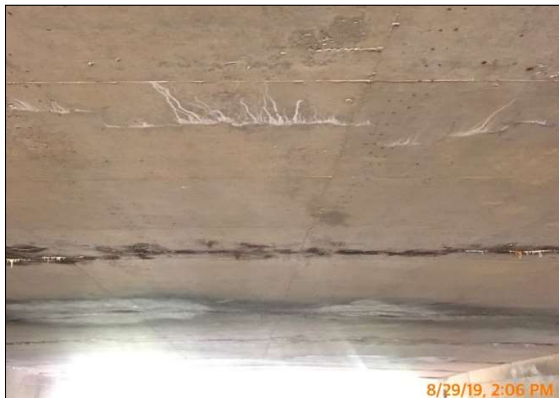
Figure 1.1.1.4-1: Example of exposure adjustment to capture details under structure, resulting in overexposed area at bottom of photo. Better framing to avoid outside area or changing direction photo is taken would improve photo.
