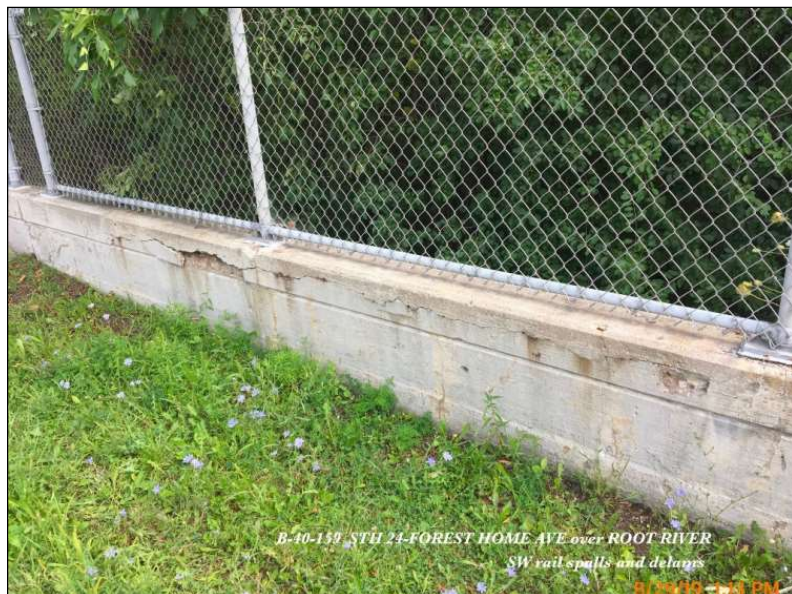
Figure 1.1.1.5-6: Same wall from medium angle clearly shows extent of defect
