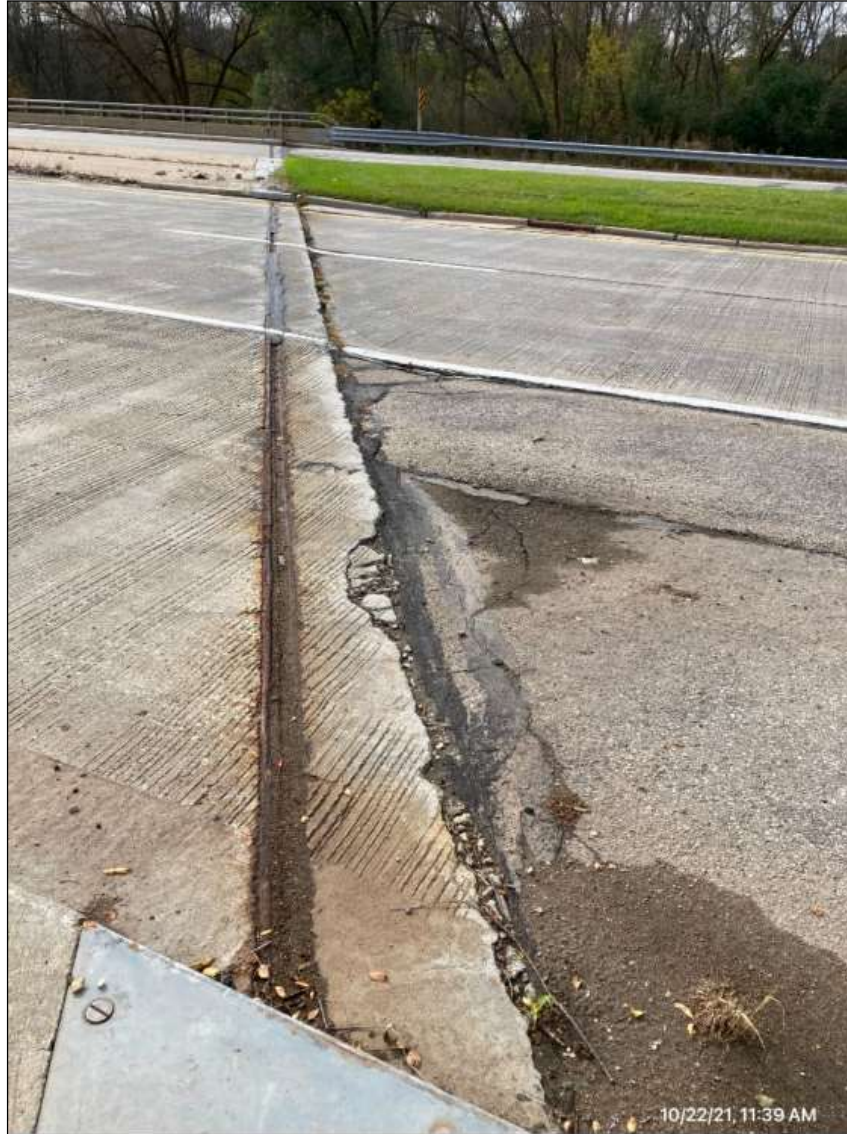
Figure 1.1.1.6-1: Good maintenance photo showing damage, location, and extent of header damage in shoulder. Provide notes to support photo. For repair of asphalt paving, additional photos of extents would be useful.
