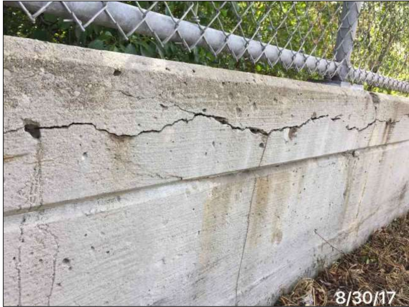
Figure 1.1.1.5-7: Too close and angled doesn't show extent of defect. Useful if included and labeled with one of the above photos
