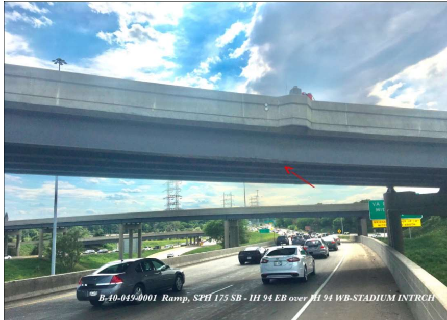
Figure 1.1.1.6-2: Photo showing location of damage in context of roadway. From this, right lane and shoulder closure would be required to repair the area with the arrow. Additional closer photos also would be required. Ideally this would be taken at an angle that clearly shows position relative to lane, but traffic did not allow.
