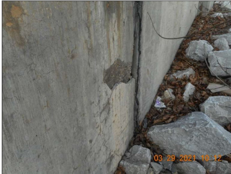
Figure 1.1.1.5-3: Good scale on photo: Leaves, riprap, trash present for scale, taken at angle that shows size of spall and offset of joint
