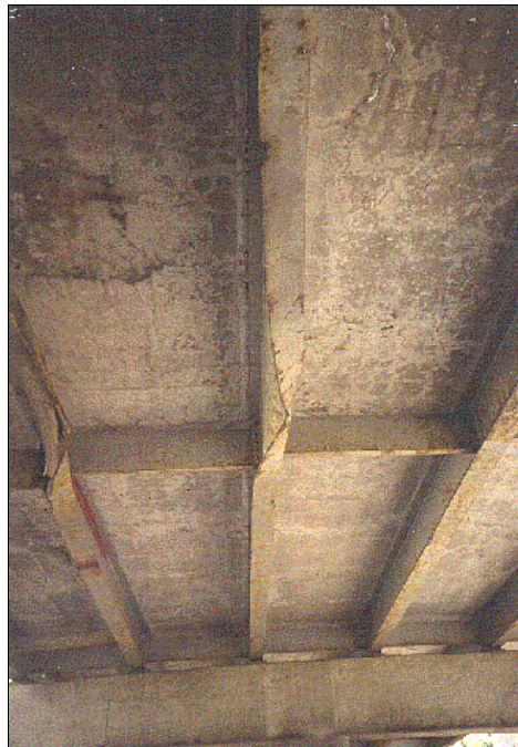
Figure 1.3.12.1-1: Impact Damage to a Steel Girder Bridge.
