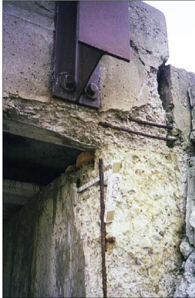
Figure 1.3.11.1-1: Tendon Section Loss at the Bottom of a Prestressed Channel and Pier Section Loss.
