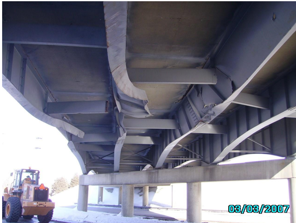
Figure 1.3.16.1-1: Critical Finding Photo
