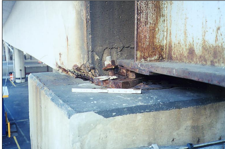
Figure 1.4.3.3-2: Failed Bearing at Pier.
