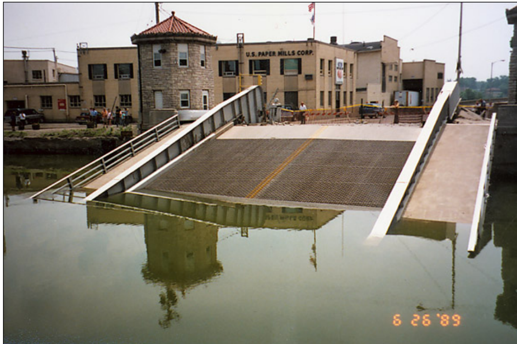
Figure 1.4.2.1-1: Failed Tayco Street Bascule Bridge, Menasha.
