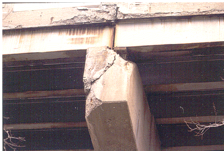
Figure 1.4.3.3-3: Damage Resulting From Failed Joint.
