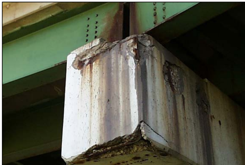
Figure 2.1.4.1-6: Spalled Concrete on Pier Cap.
