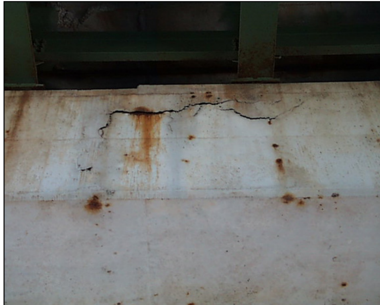
Figure 2.1.4.1-5: Delaminations on Concrete Pier.
