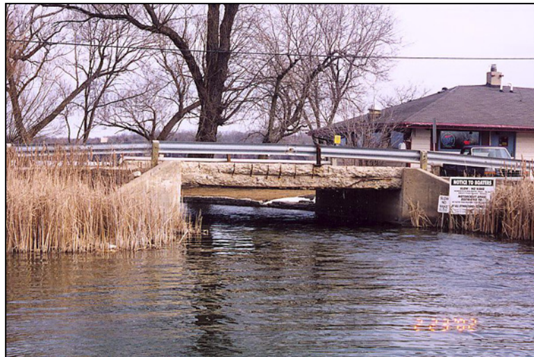
Figure 2.1.5.1-1: Heavily Deteriorated Single Span Concrete Slab.
