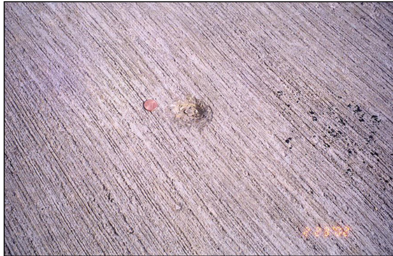
Figure 2.1.4.1-10: Pop-out on Concrete Deck.
