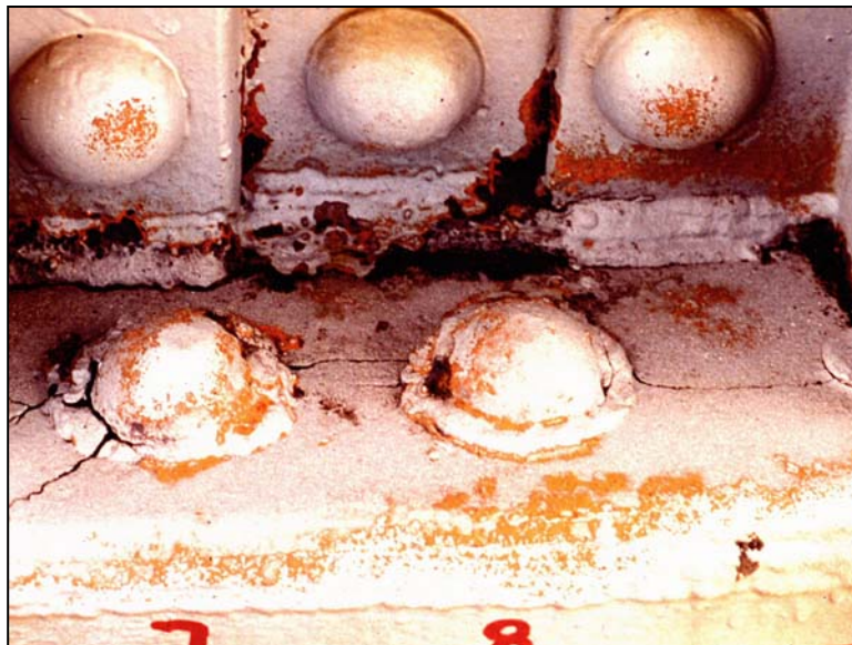
Figure 2.1.4.4-4: Fatigue Cracks on a Steel Casting.
