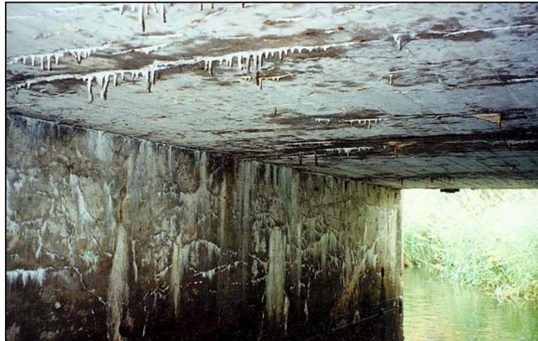
Figure 2.1.4.1-8: Heavy Efflorescence on an Abutment and Slab.
