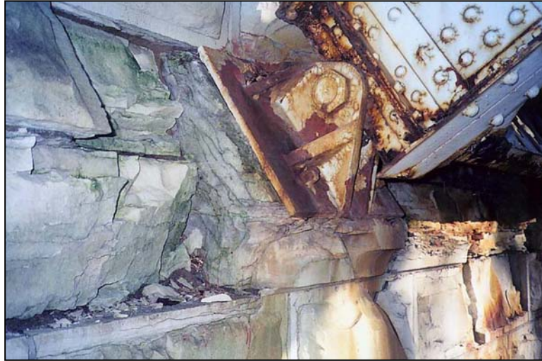
Figure 2.1.4.4-1: Masonry Deterioration/Spalls at an Arch Bearing.
