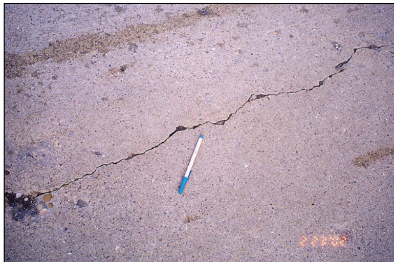
Figure 2.1.4.1-2: Medium Longitudinal Crack in a Concrete Deck.
