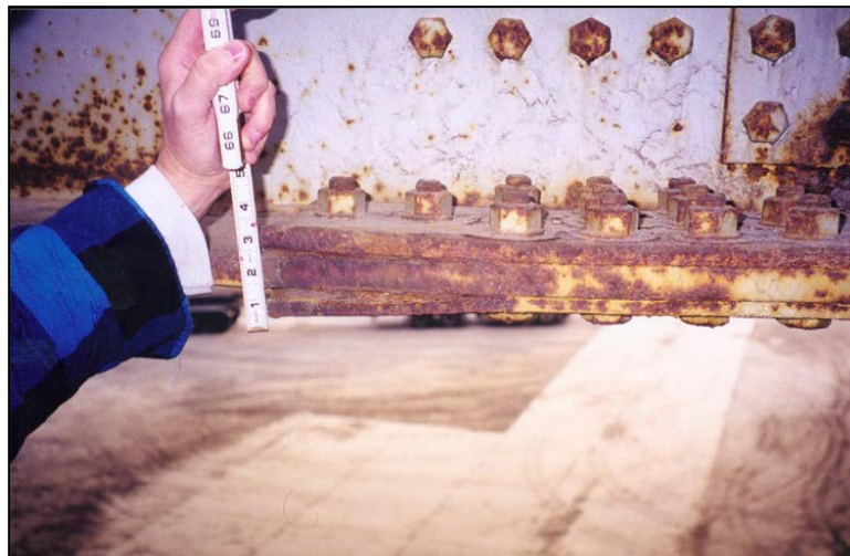
Figure 2.1.4.2-7: Pack Rust Prying Apart Flange Splice Plates.
