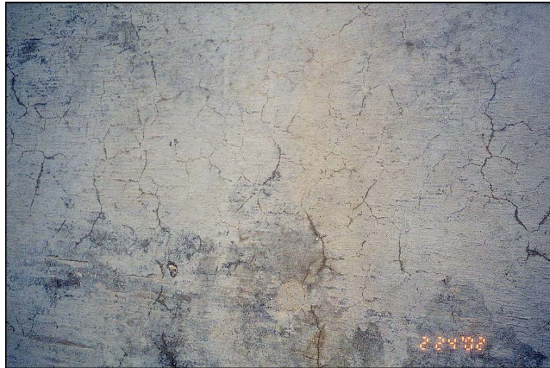
Figure 2.1.4.1-1: Map Cracking in Reinforced Concrete.
