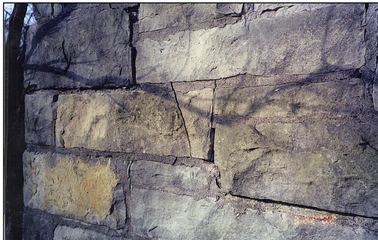
Figure 2.1.4.4-2: Split Masonry Unit with Failing Mortar Joints.
