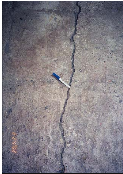
Figure 2.1.4.1-3: Wide Vertical Crack in an Abutment.
