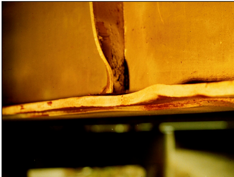
Figure 2.1.4.2-8: Girder Bottom Flange Impact Damage.
