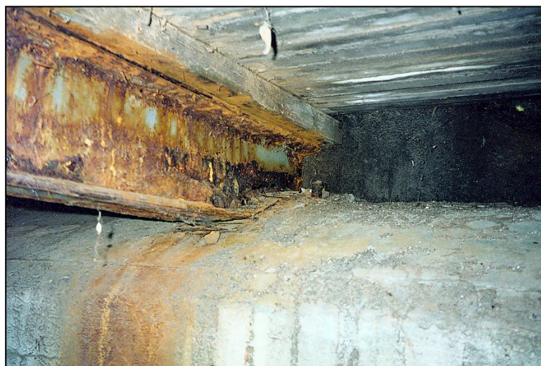
Figure 2.1.4.2-6: Corrosion and Loss of Section - Crushed Beam at Abutment.
