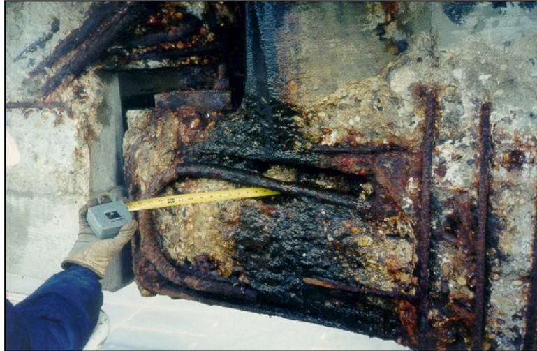
Figure 2.1.4.1-7: Reinforcing Steel Corrosion.
