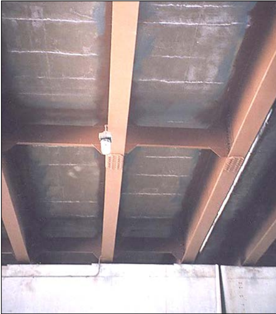
Figure 2.3.2.1-2: Cracking of Concrete Deck (Localized Area Over Pier) – Condition State 2.
