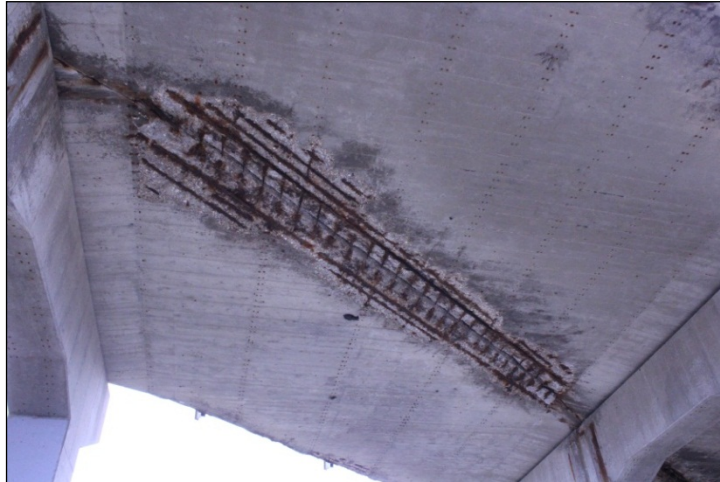
Figure 2.3.2.1-1: Reinforced Concrete Slab w/ Spalling and Exposed Corroded Reinforcing - Condition State 3.
