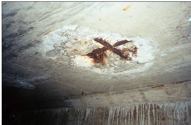
Figure 2.3.3.2-1: Localized Spall with Exposed/Corroding Rebar on the Deck Underside of a Post-Tensioned Box Girder.
