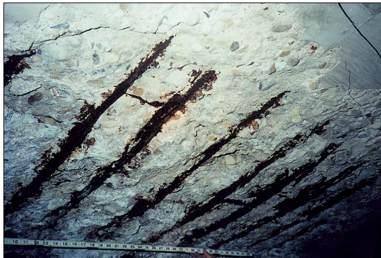
Figure 2.3.2.2-2: Reinforced Concrete Box Girder Top Flange/Deck Localized Rebar Corrosion and Bond Loss.
