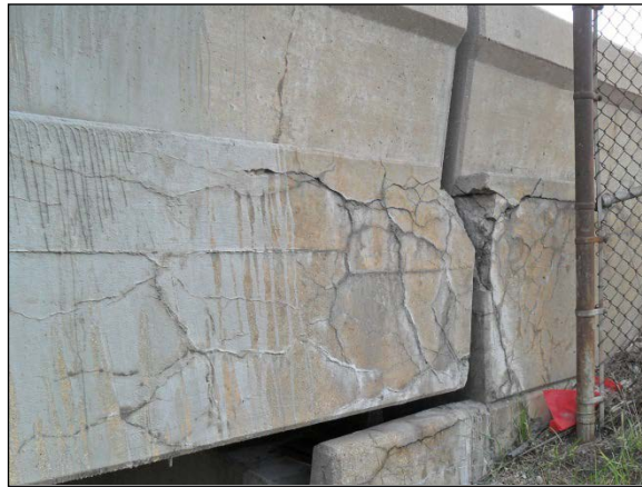
Figure 2.3.2.1-4: Typical Reinforced Concrete Slab Distress.
