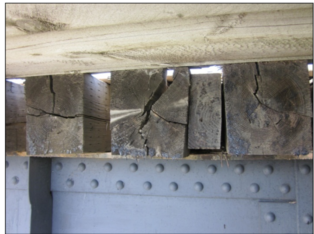
Figure 2.3.5.1-3: Timber Deck (Railroad Ties) – Condition State 3.
