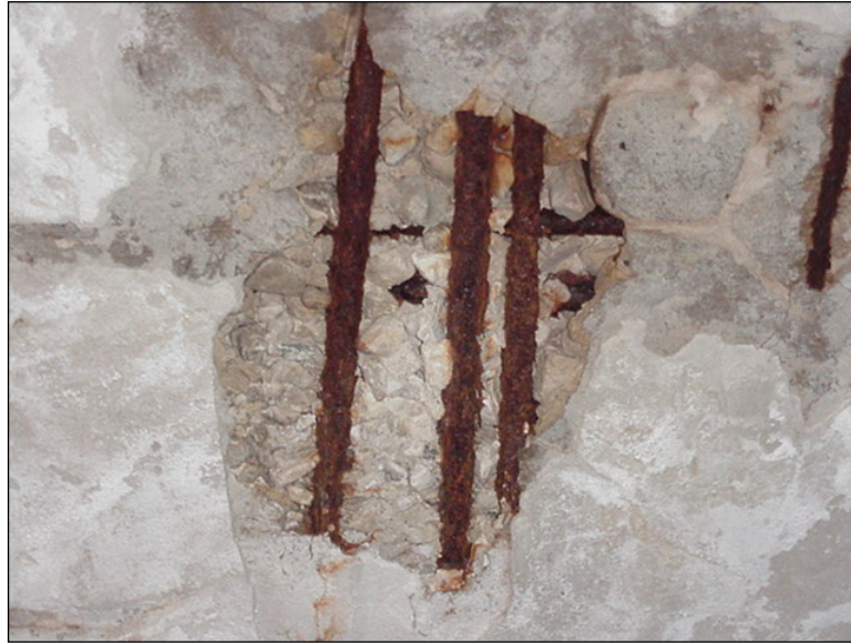
Figure 4.4.2-22: Concrete Spalling with Exposed Reinforcing Steel.
