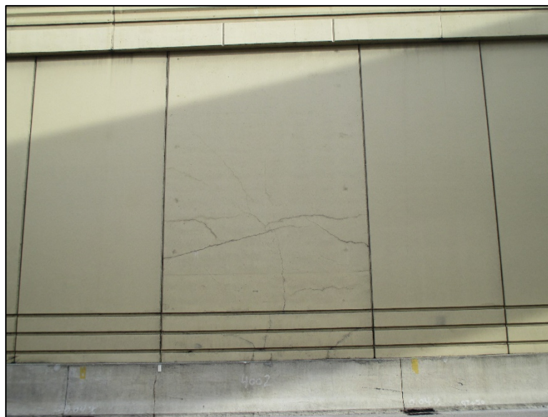
Figure 4.4.4-16: Excessive Cracking within Secant Wall Facade Concrete Panel.
