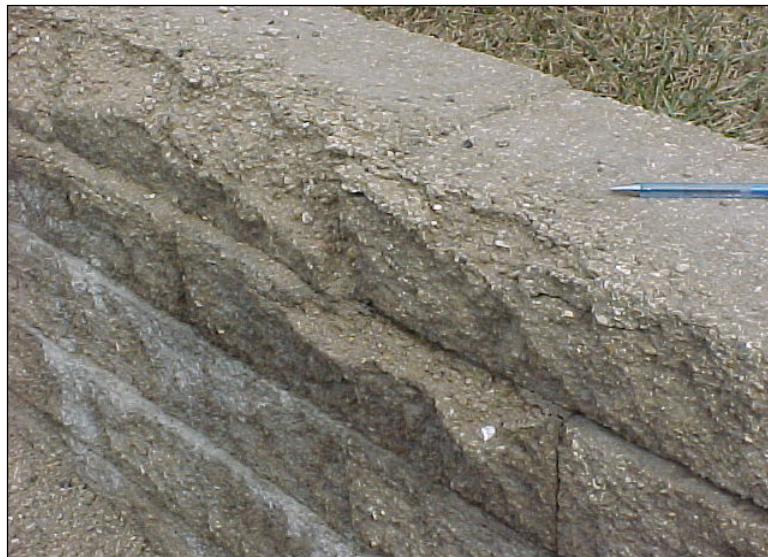
Figure 4.4.2-17: Spalling and Fraying on the Top Edge of the Block.
