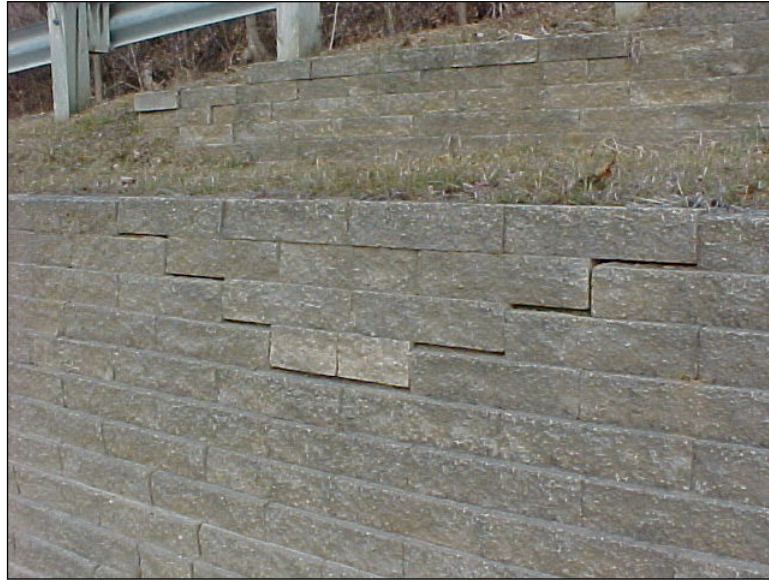
Figure 4.4.2-13: Poor Construction Methods Resulting in Block Separation.
