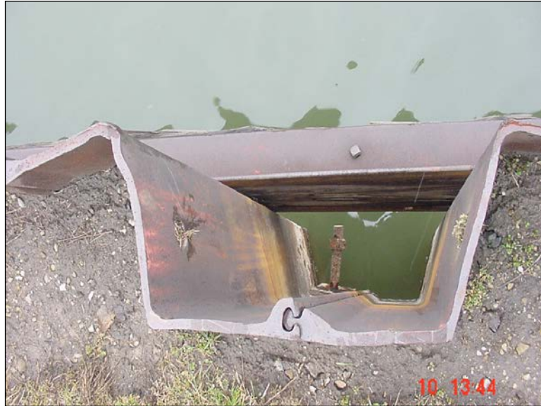
Figure 4.4.4-12: Failed Tie-rod Along a Sheet Pile Dockwall.
