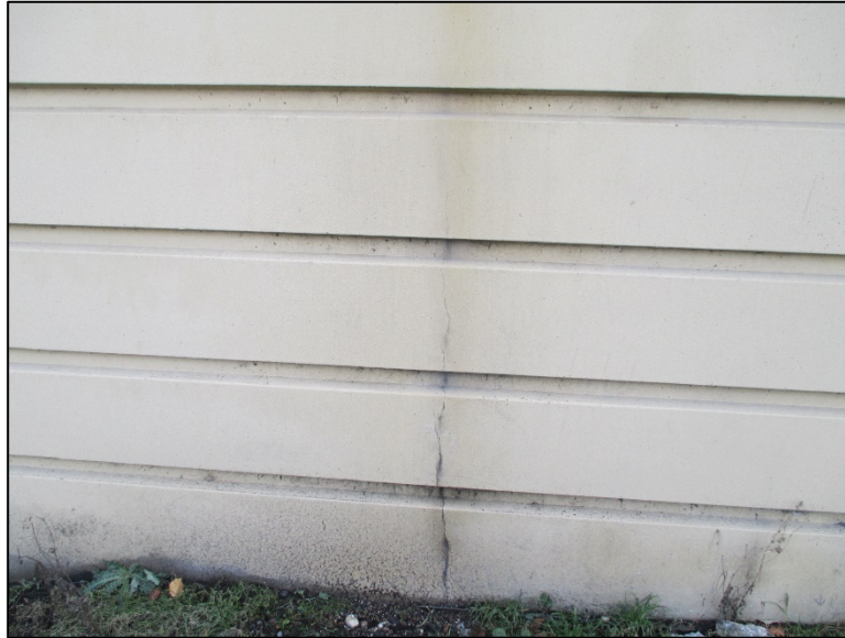
Figure 4.4.2-21: Vertical Crack Through Precast Concrete Panel.
