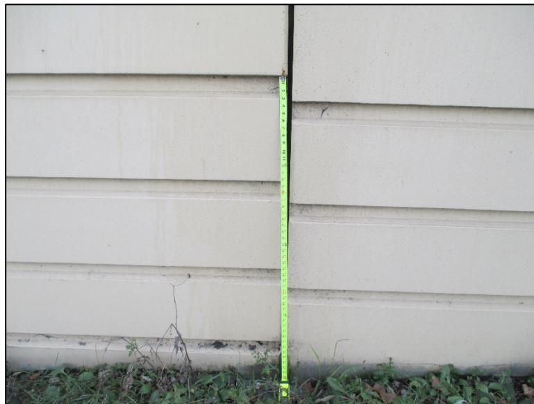
Figure 4.4.2-8: View of Differential Settlement between Precast Concrete Panels. Note Misalignment in Rustication.
