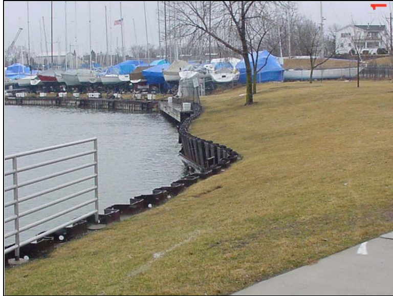
Figure 4.4.4-11: Tilted and Deformed Sheet pile Dockwall.
