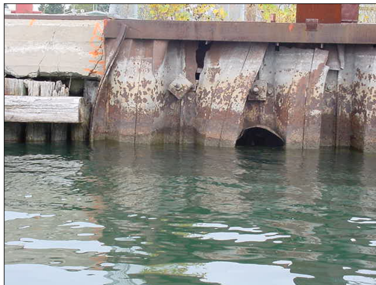
Figure 4.4.2-1: Impact Damage to a Steel Sheet Pile Dockwall.
