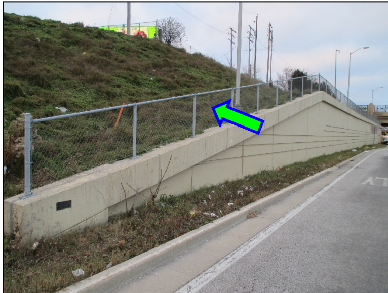
Figure 4.4.5-8: Protective Screening Fastened to a Horizontal Coping. Note the Screening is Not Adjacent to a Sidewalk.
