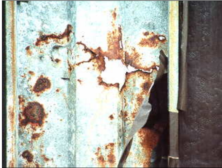
Figure 4.4.2-23: Severely Corroded Steel Sheeting Cantilever Wall.
