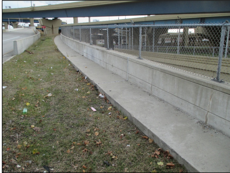
Figure 4.4.5-13: Drainage System Along Top of Retaining Wall. Note Vegetation Exhibits No Signs of Erosion or Settlement.
