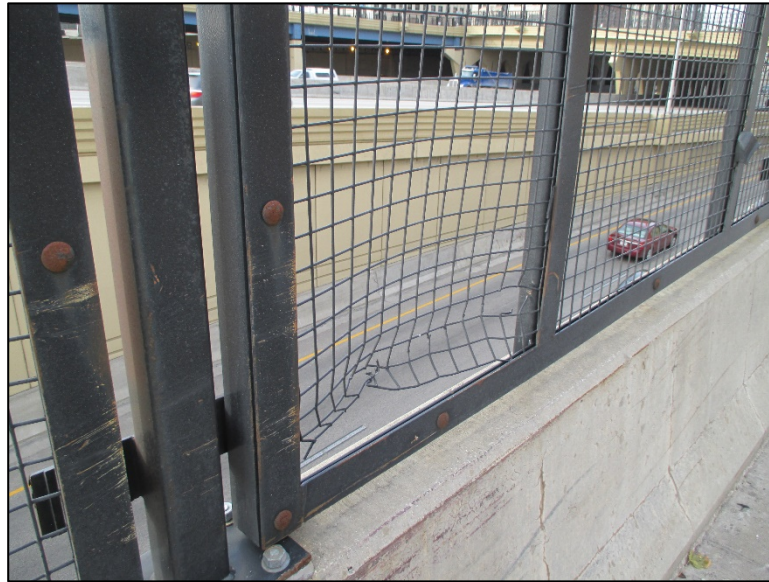
Figure 4.4.5-9: Assessment State 3 Protective Screening atop Bridge Rail. Note Chain-link Fence Deformation but Function Remains.
