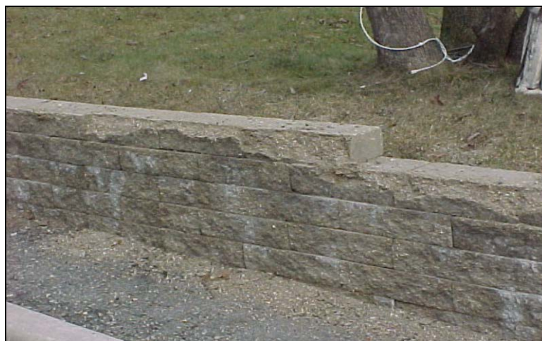
Figure 4.4.2-16: White Precipitate Formed due to Efflorescence.
