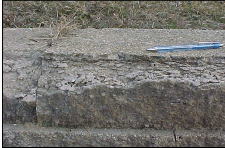
Figure 4.4.2-18: Freeze-Thaw Damage at a Corner.
