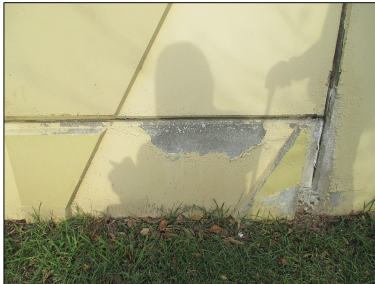
Figure 4.4.5-2: Failed Concrete Stain.
