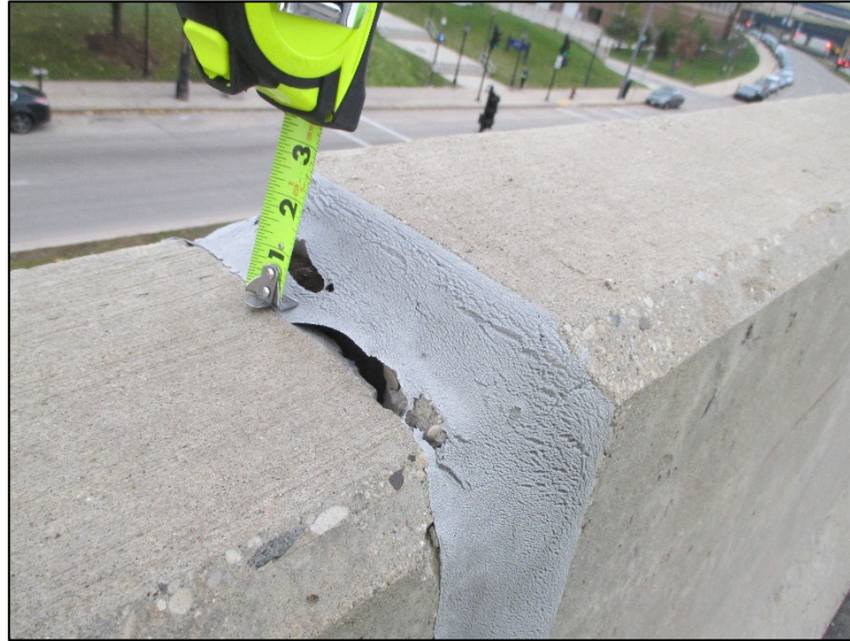
Figure 4.4.2-9: Settlement as Seen from Bridge Rail at Top of Wall. Note, Settlement was Reflected in Adjacent HMA Pavement.
