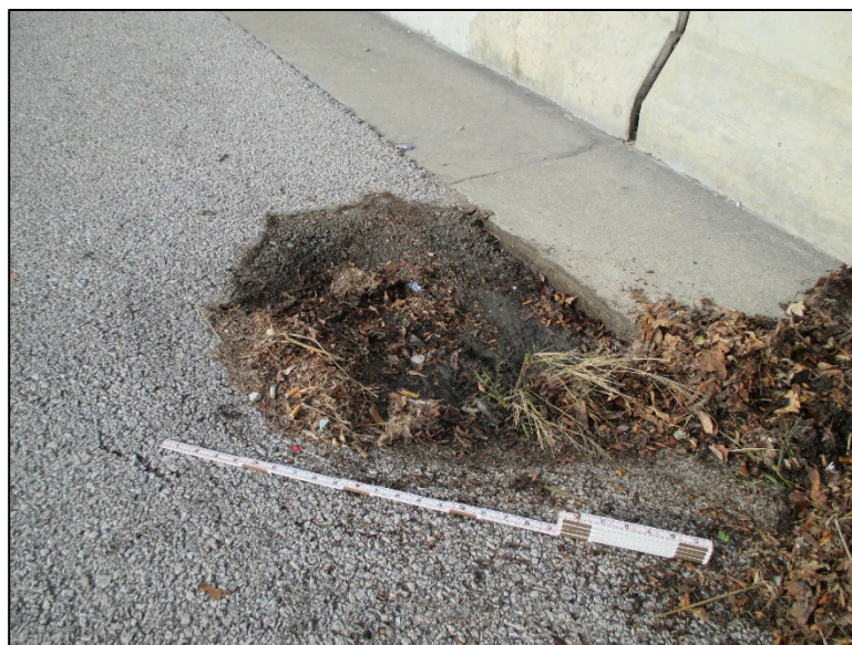
Figure 4.4.5-12: Pothole Due to Loss of Fill Within Shoulder Gutter Pan Along Top of Retaining Wall.
