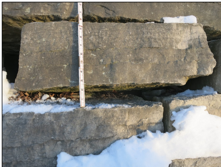
Figure 4.4.2-20: Excessive Gap Forming At Base of Stone Block.
