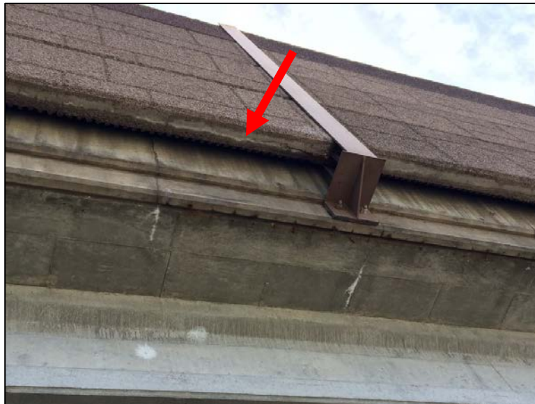
Figure 4.5.4-8: Cracking with Efflorescence Along Midline of Underside Panel.
