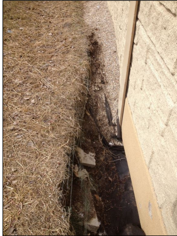
Figure 4.5.5-2: Drain tile system failure below noise wall resulting in loss of material and exposure of noise wall footing.
