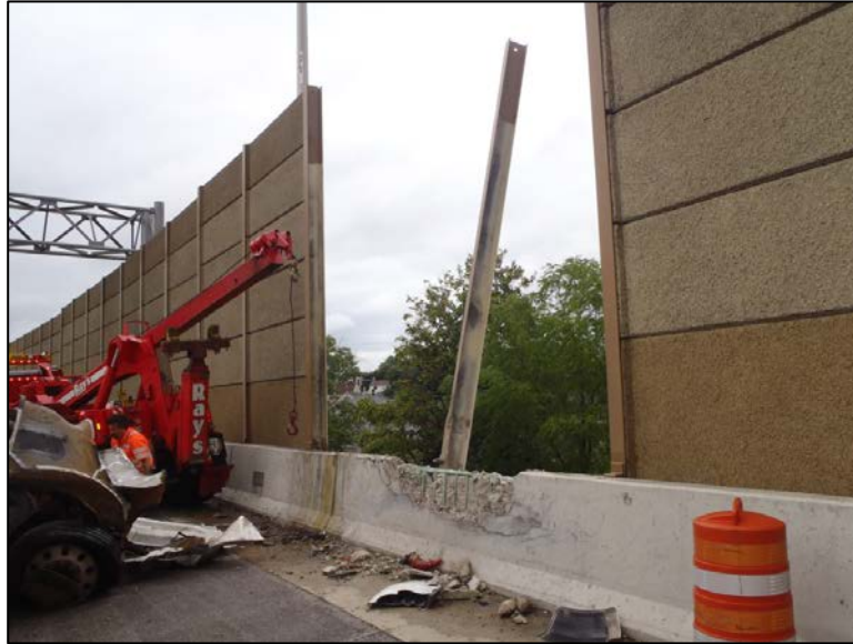
Figure 4.5.4-3: Impact Damage with Failed Post and Paneling of Structure Mounted Noise Wall.
