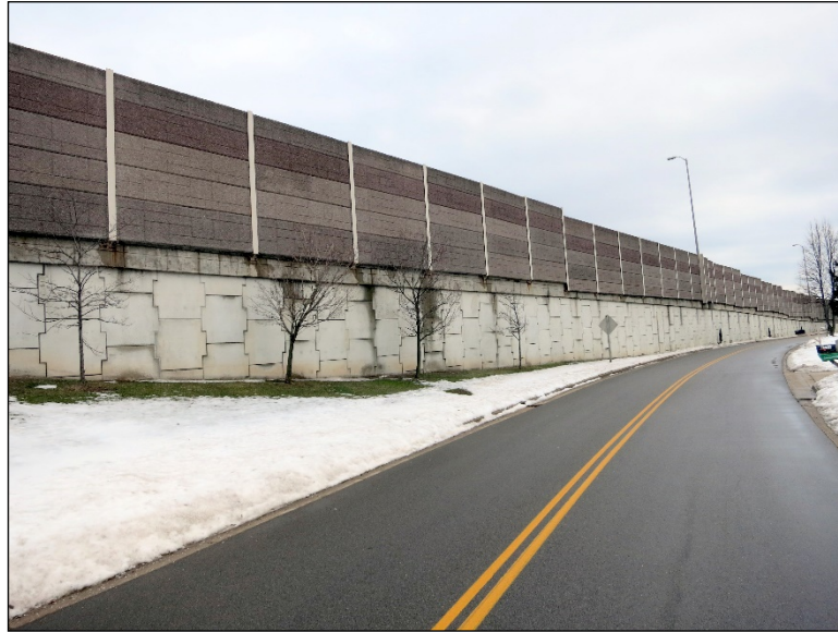
Figure 4.5.1-5: Precast Concrete Panel Noise Barrier Wall Mounted on a Retaining Wall.
