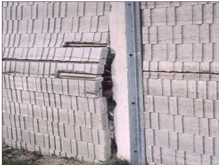
Figure 4.5.5-1: Lateral Movement of a Noise Barrier Wall.
