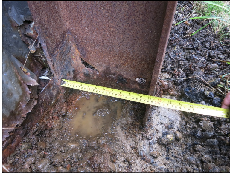
Figure 4.5.4-13: View of Through Section Loss Along the Base of a Post for a Post and Panel Noise Wall.
