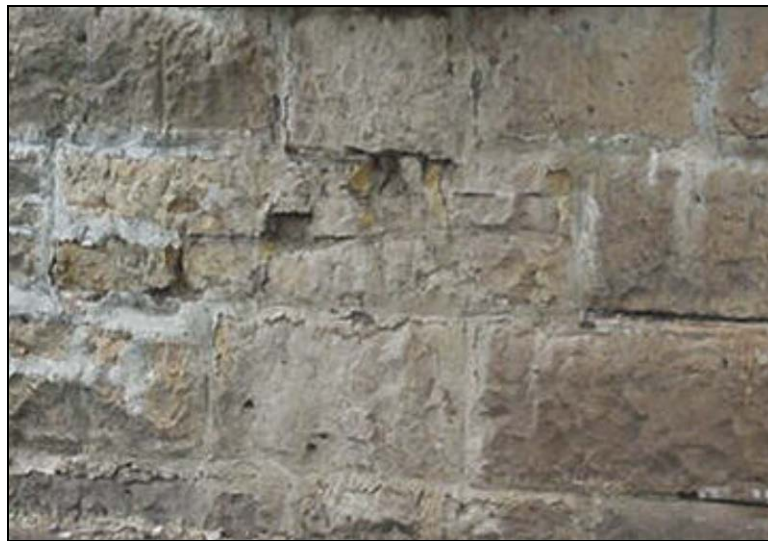
Figure 4.5.4-5: Heavy Scaling with Efflorescence on a Masonry Noise Barrier Wall.
