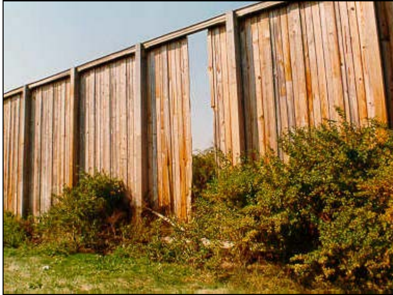
Figure 4.5.4-10: View of Broken and Missing Timber Planks.
