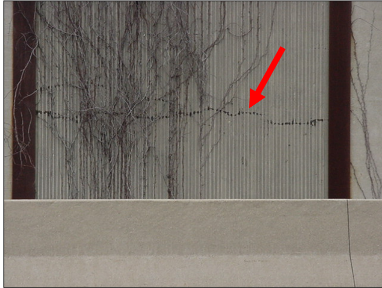
Figure 4.5.4-7: Concrete Panel Noise Barrier Wall with a Horizontal Crack at Mid-Panel.
