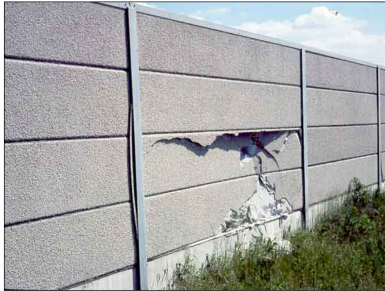
Figure 4.5.4-1: Impact Damage to a Noise Barrier Wall.
