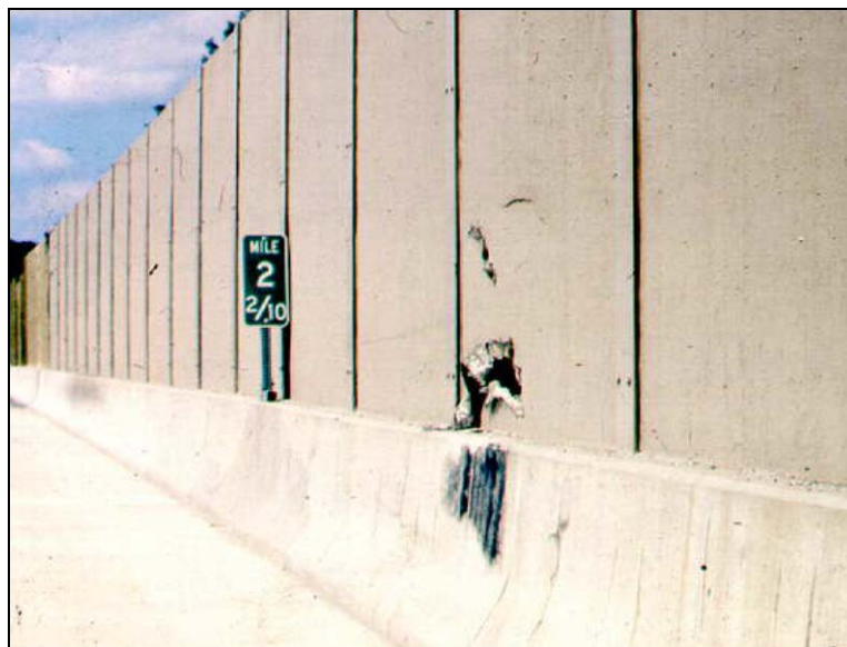
Figure 4.5.4-2: Impact Damage to a Noise Barrier Wall.
