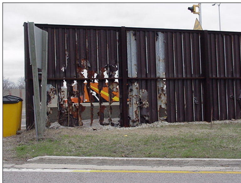
Figure 4.5.4-12: Severe Corrosion of a Metal Noise Barrier Wall.
