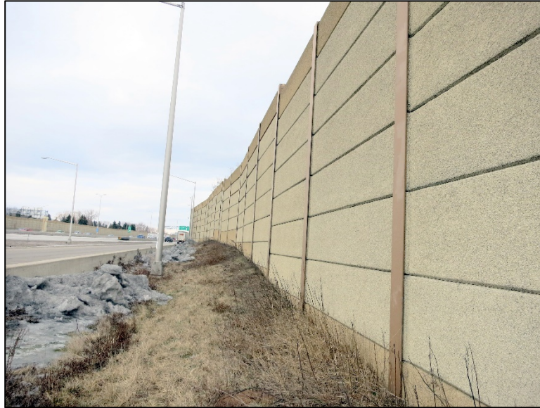
Figure 4.5.4-6: Overall View of a Concrete Noise Barrier Wall Comprised of Reinforced Concrete Core and Durisol (wood/cement fiber) Cladding.
