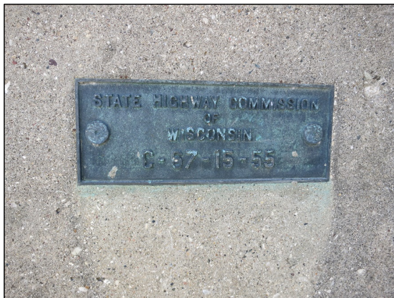
Figure 4.6.3-1: View of Name ID Plaque located on the Wing of a Culvert End Treatment.
