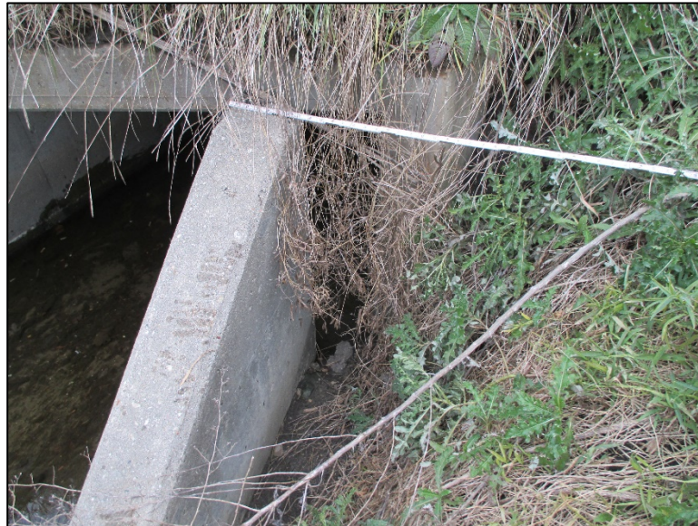
Figure 4.6.6-14: View of Wingwall Movement. Note loss of fill behind wingwall and culvert barrel – Condition State 3.
