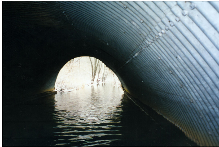
Figure 4.6.6-5: Severely distorted barrel – Distortion Condition State 4.
