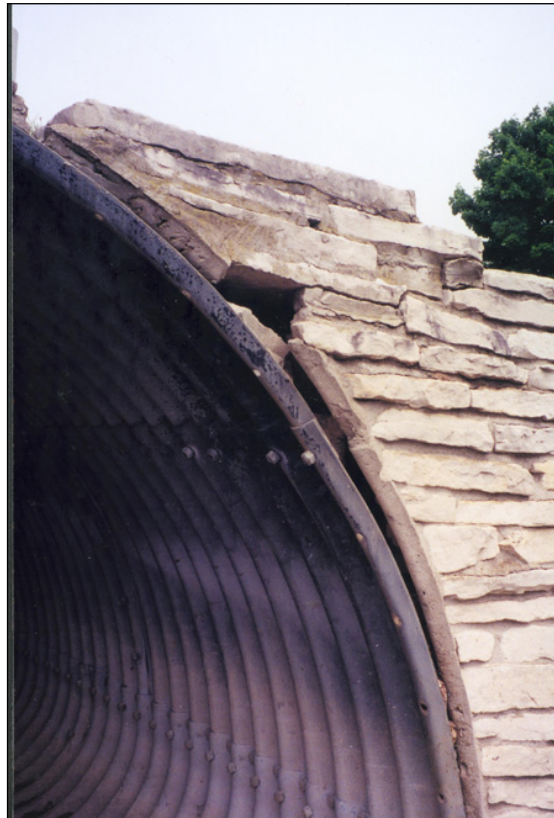
Figure 4.6.7-2: Masonry headwall separating from the barrel.
