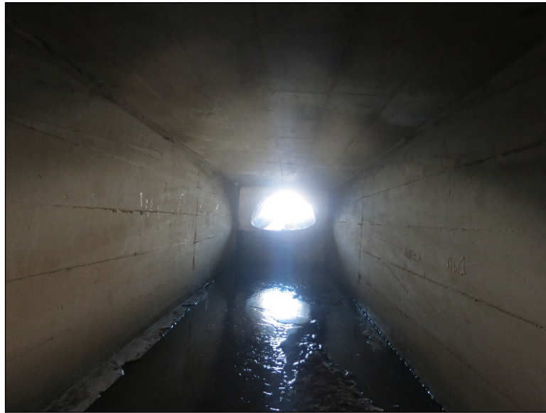
Figure 4.6.4-5: View of reinforced concrete single cell box culvert with corrugated steel pipe arch extension
