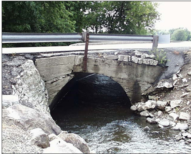
Figure 4.6.7-1: Concrete headwall failure. Note: Headwall deterioration would be captured under Assessment 9248 – Culvert End Treatment
