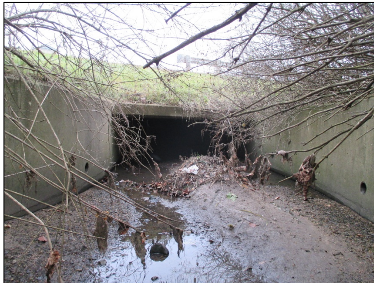
Figure 4.6.6-13: View of Retaining walls extending beyond limits of integral wingwalls.
