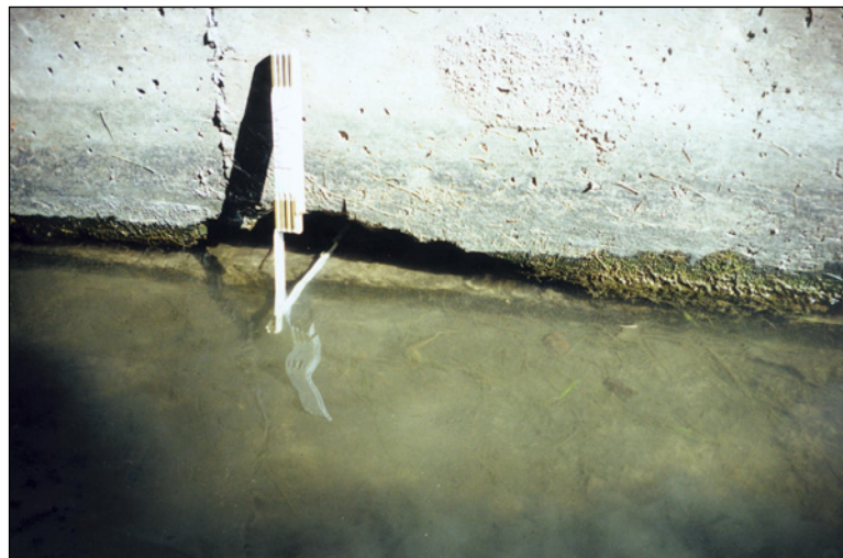
Figure 4.6.7-3: Through thickness section loss at water line of wall separating two cells.
