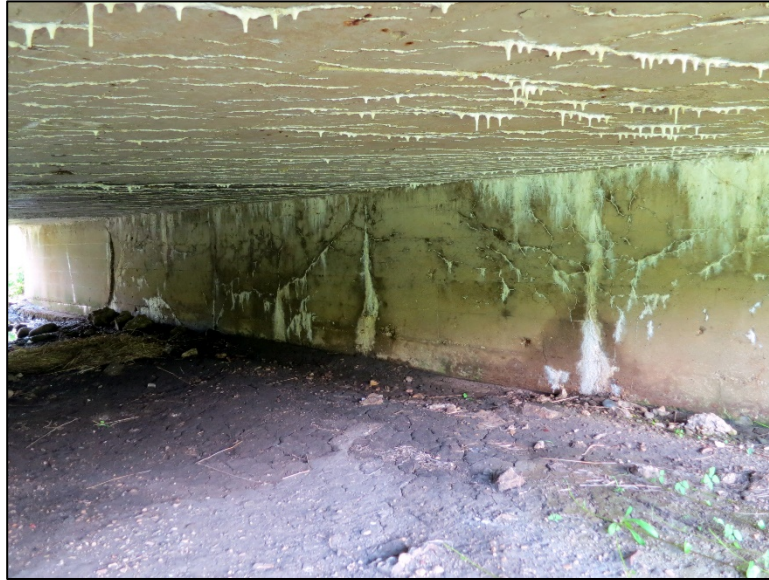
Figure 4.6.6-7: Deterioration on Culvert Wall – Heavy Density Cracking with Efflorescence Condition State 4.
