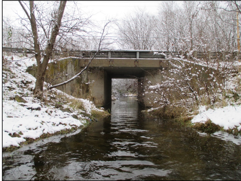
Figure 4.6.3-2: A bridge like structure with total length less than 20 ft. This structure is designated as a small bridge in HSI, and inspected with bridge elements.
