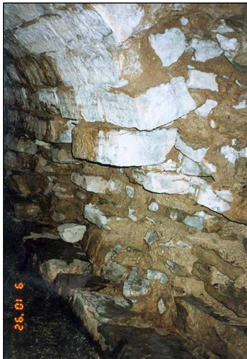
Figure 4.6.6-10: Masonry Culvert with Severe Deterioration of Mortar Joints.
