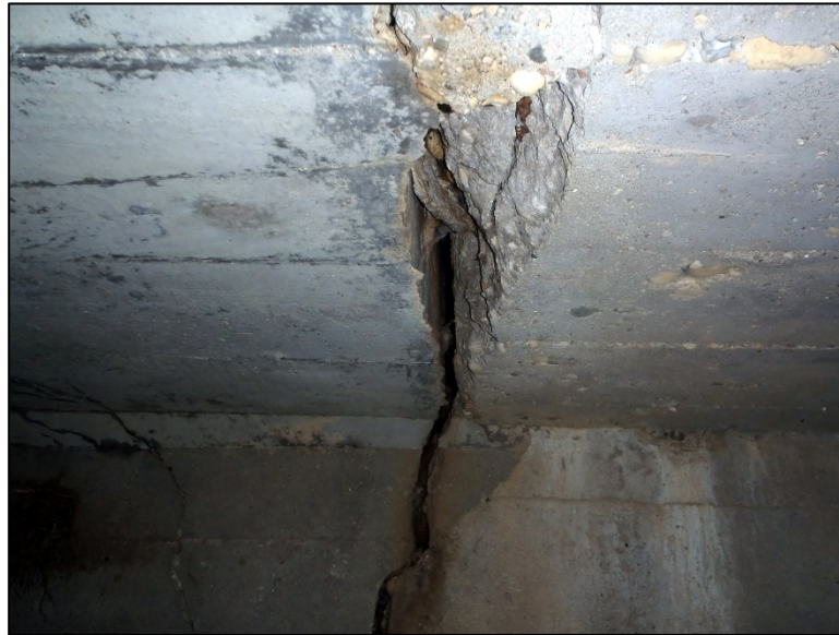
Figure 4.6.6-9: Joint Separation Between Pipe Segments – Settlement Condition State 3.
