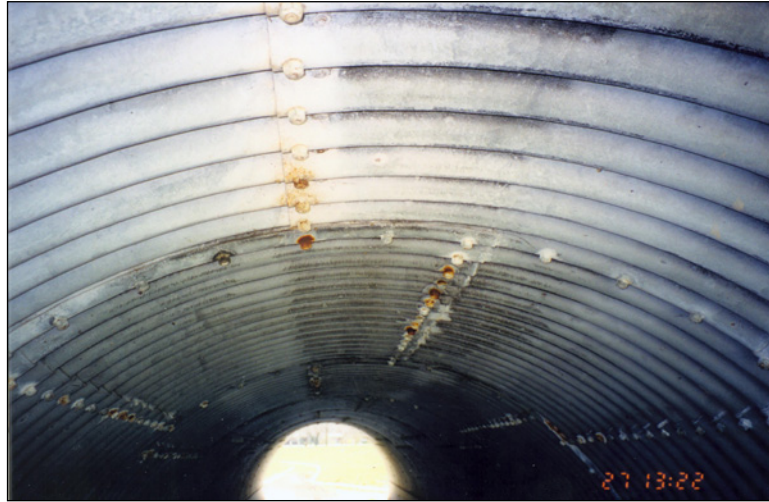
Figure 4.6.6-3: Light to moderate bolt corrosion – Connection Condition State 2.
