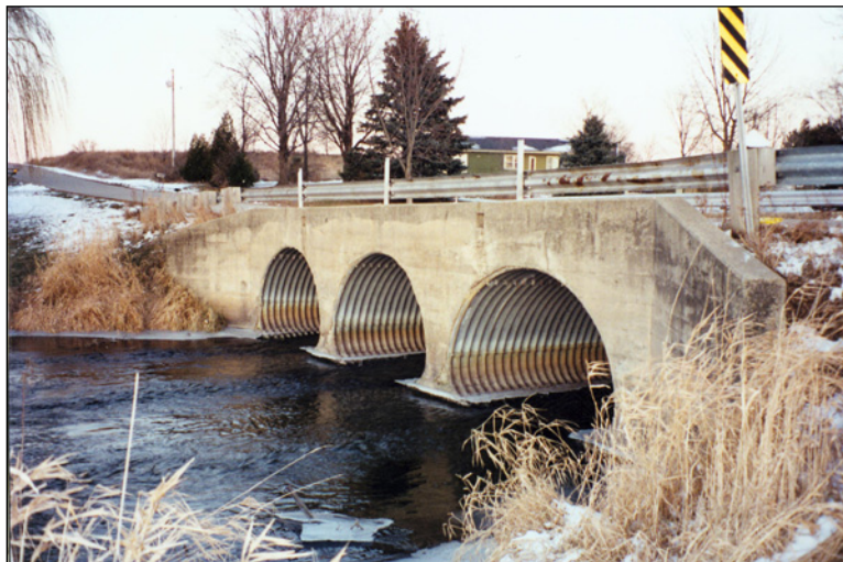
Figure 4.6.6-2: Surface corrosion near the waterline – Corrosion Condition State 2.
