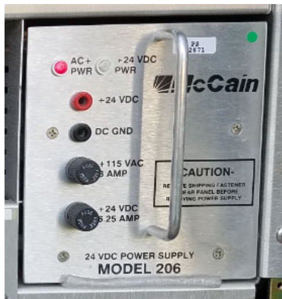
Power Source (bottom section of cabinet)
