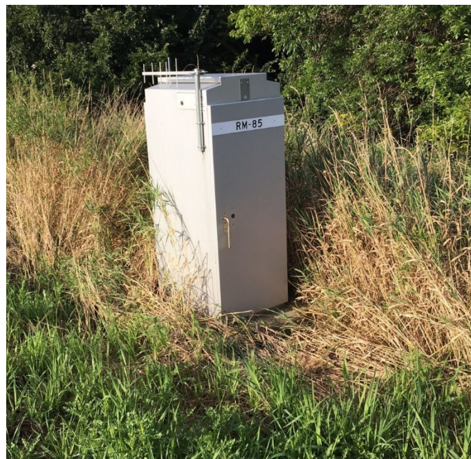
Figure 3.3.6 Exterior of Cabinet
