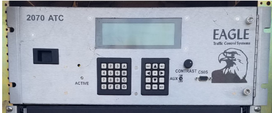
Type 2070 Signal Controller (upper section of cabinet)
