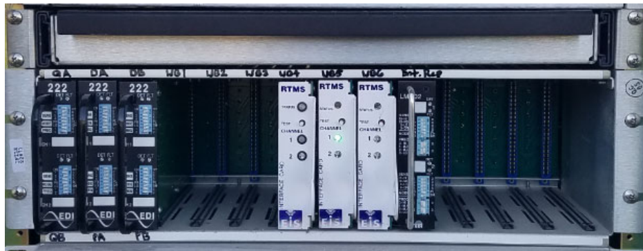
Detectors Amplifiers (middle section of cabinet)
