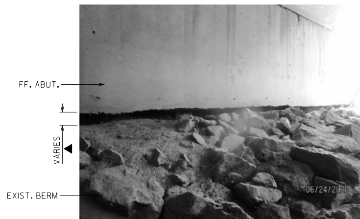
UNDERMINING AT B-11-137 N. ABUT.
