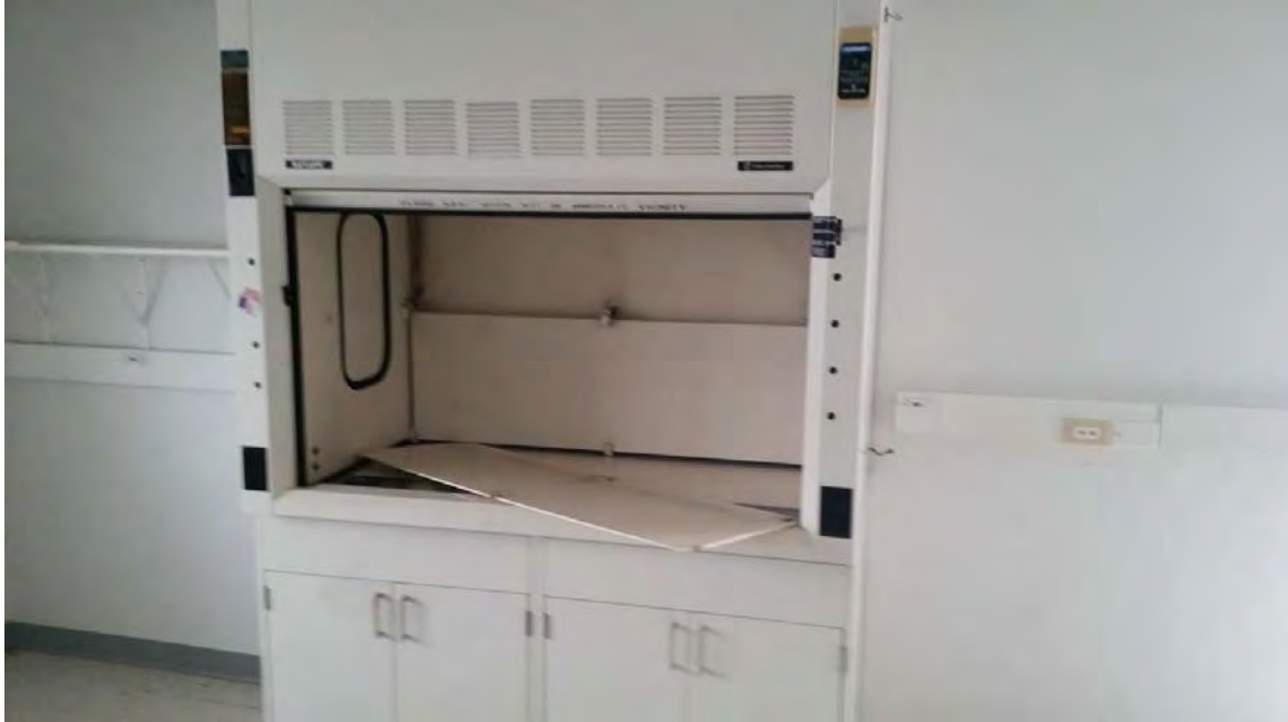
Fume Hood in Lab Room
